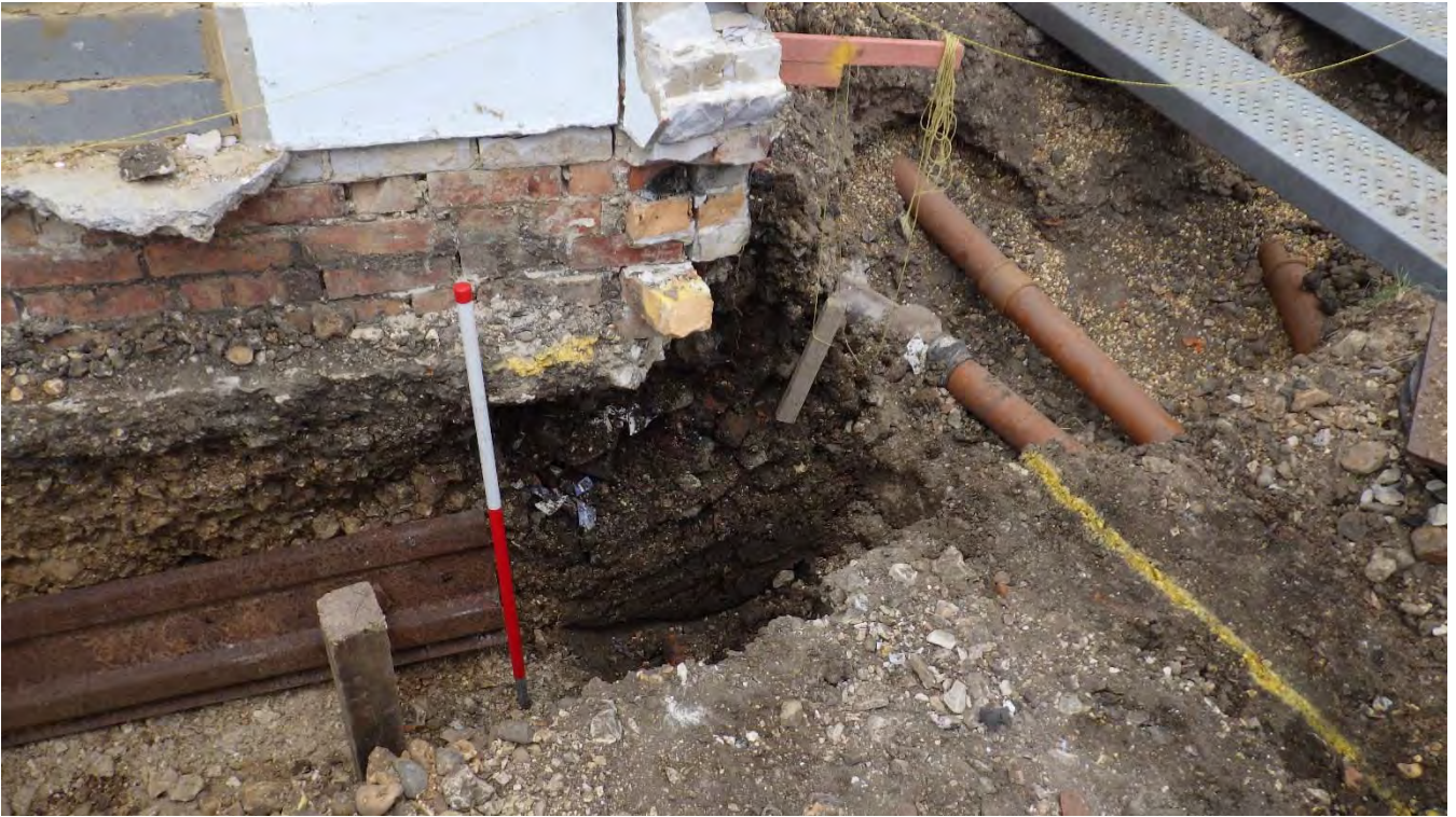
Plate 3: F102 in section with concrete platform of building above it. View from the south. Scale 1m
