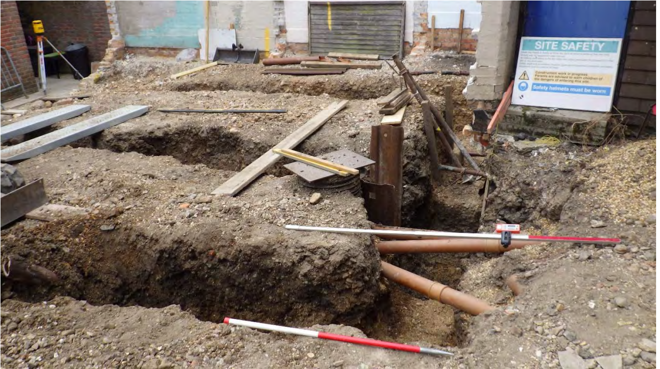
Plate 1: The site during excavation of building footings. View from the east. Scale 1m
