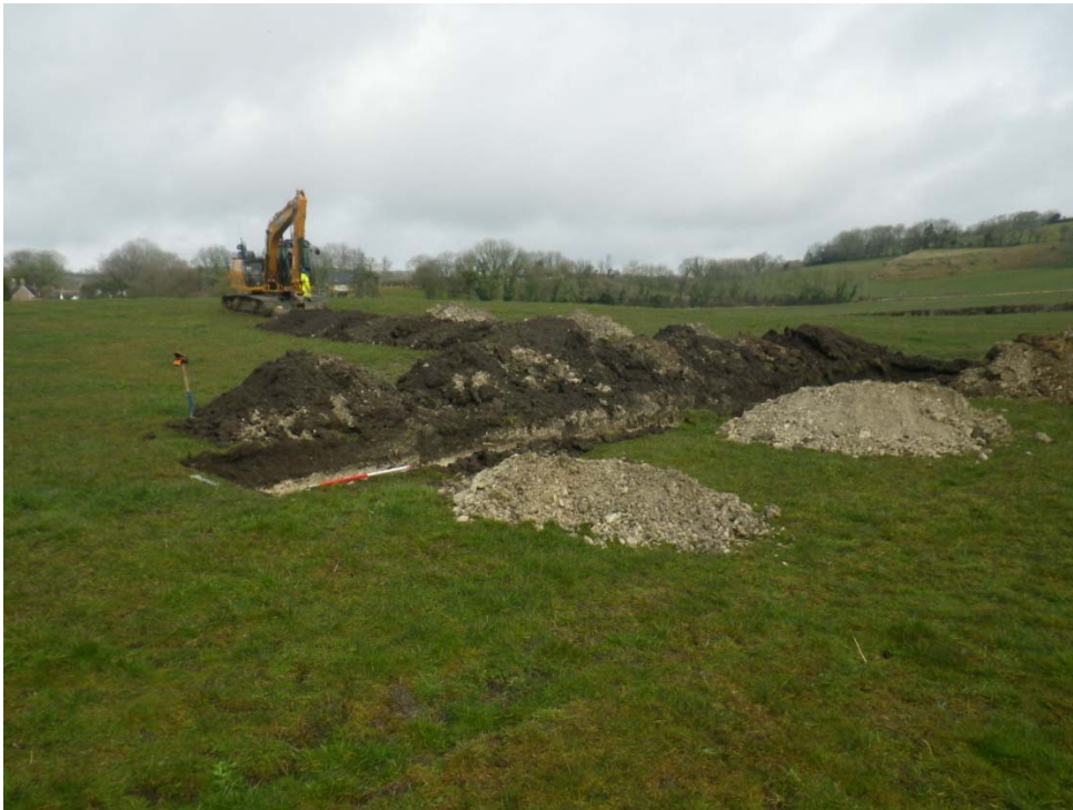
Plate 1: View of excavated trenches and site setting. View from the south-east. Scale 1m
