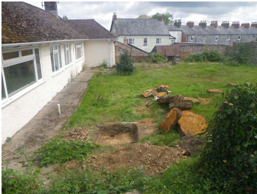
Location of trial pit within footprint of proposed extension. View from west
