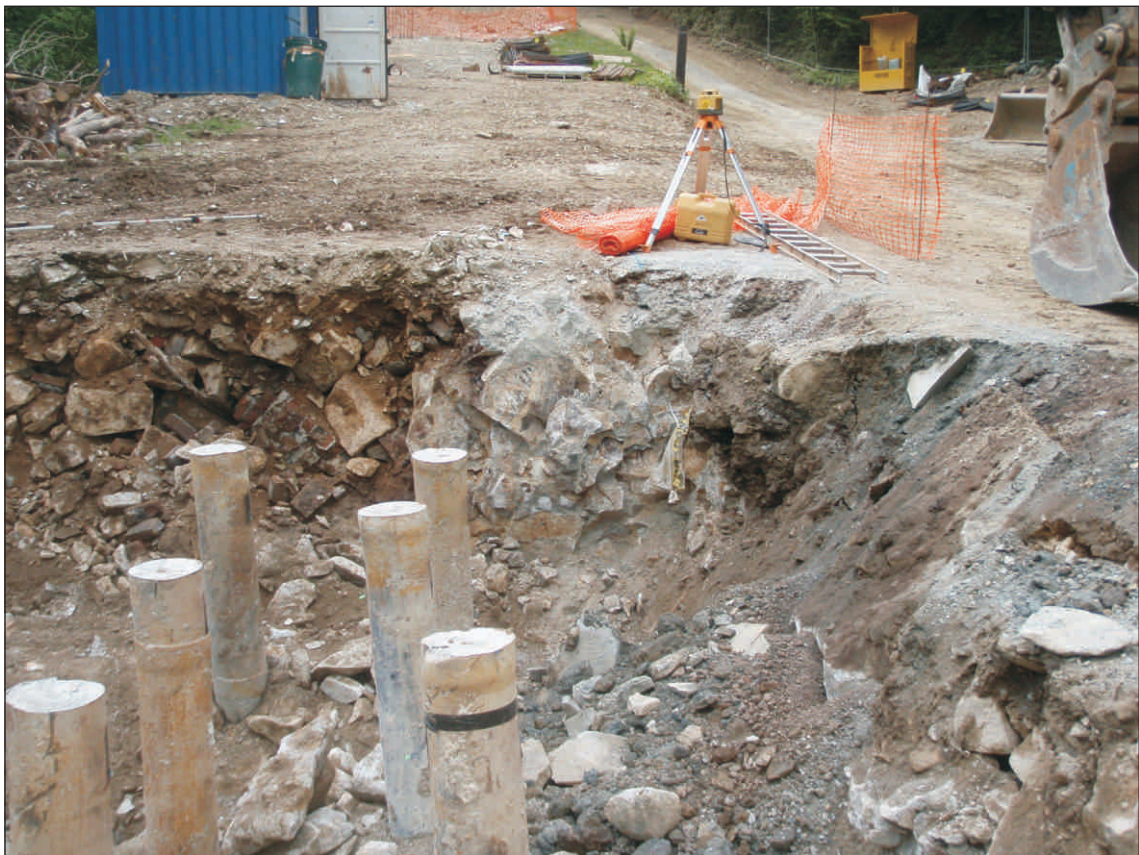
Plate 2: Remains of original viaduct pier base in Pier C excavation, view to north.
