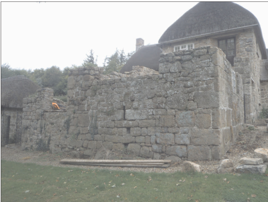
Plate 2: The south elevation of the shippon showing drain outlets and vent, with the outshut to the left, viewed from the southeast
