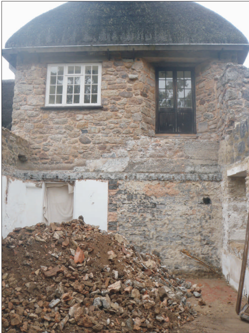
Plate 3: The east end of the shippon showing the gable wall of the farmhouse with C20 ground-floor wall, viewed from the south
