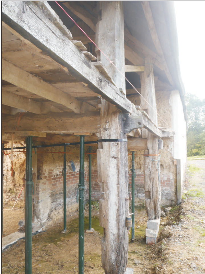
Plate 5: Type B posts in the north-west elevation, also showing pegged tongue on the first-floor beam. View from the northeast.
