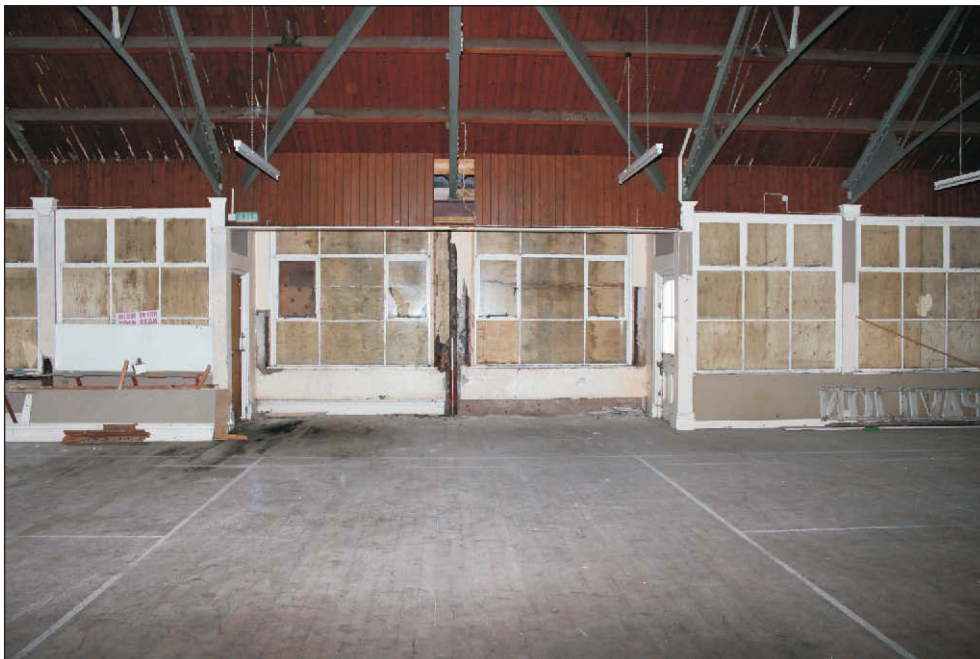
Plate 6: The first floor showing the replacement glazing in the north elevation, viewed from the south. 1m scale.
