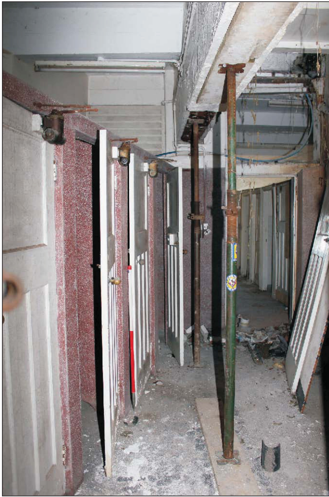
Plate 5: The ground-floor ladies' toilets showing the rear area viewed from the south. 1m scale.
