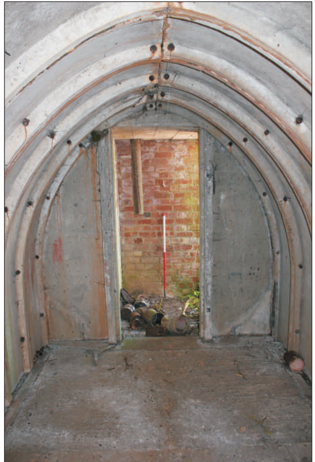
Plate 6: Pen 145, interior of air raid shelter showing pre-cast concrete construction and pipe in entranceway. View to west. 1m scale.
