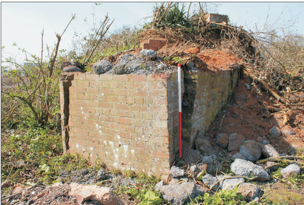
Plate 8: Pen 144, end of spine wall showing concrete filling of sandbags. View to west. 1m scale.
