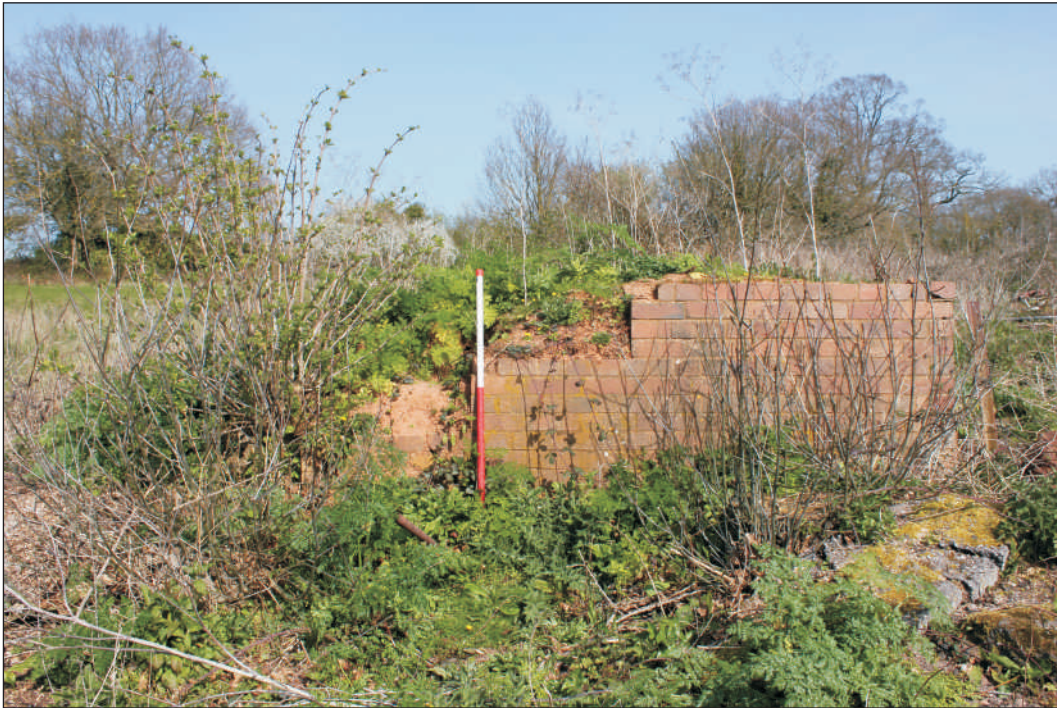
Plate 7: Pen 144, end of retaining wall showing stepped brick masonry. View to north. 1m scale.
