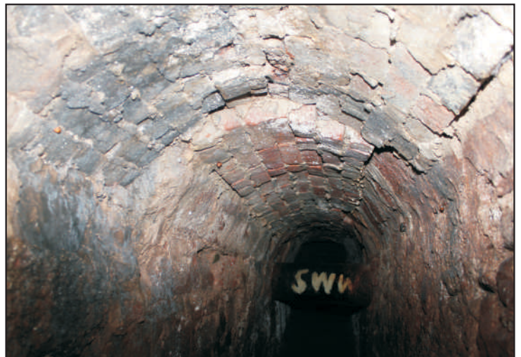
Plate 6: Brick repairs to the capping of the Cathedral Passage showing build below evaluation trench in the foreground and lower repair beyond. View to the NE
