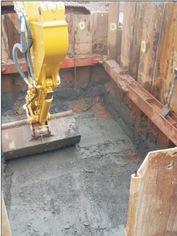
Plate 2: General view of clean alluvial clay [111] at base of launch pit looking south
