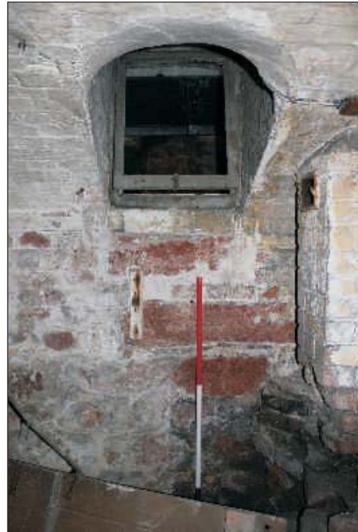
Plate 13: Coal cellar, showing vaulted ceiling, and coal chute in the east elevation, and stove viewed from the southwest. Scale 1m.
