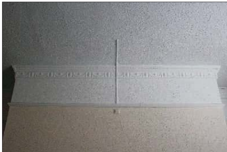
Plate 9: First floor, front room, close up of the cornice viewed from the southwest.
