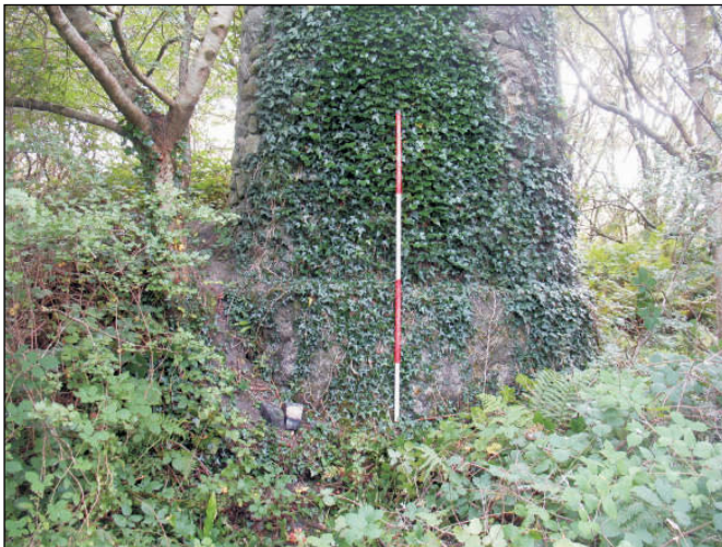
Plate 3: Molinnis chimney base showing the plinth foundation, view from northwest. Scale 2m
