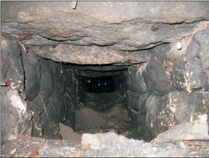
Plate 5 : Molinnis chimney flue interior, showing the stone capstones or lintels, view from west-southwest. The width of the soot-encrusted flue passage is 0.55m
