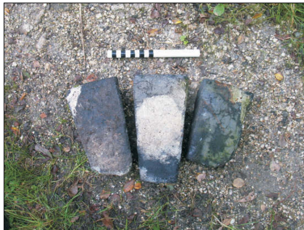
Plate 7: Examples of fallen chimney stack bricks, specially designed with a taper. Scale 0.20m
