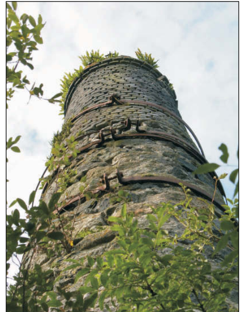
Plate 6: Molinnis chimney top, looking up from east-northeast, showing the poor state of the brickwork and the slipping iron bands.
