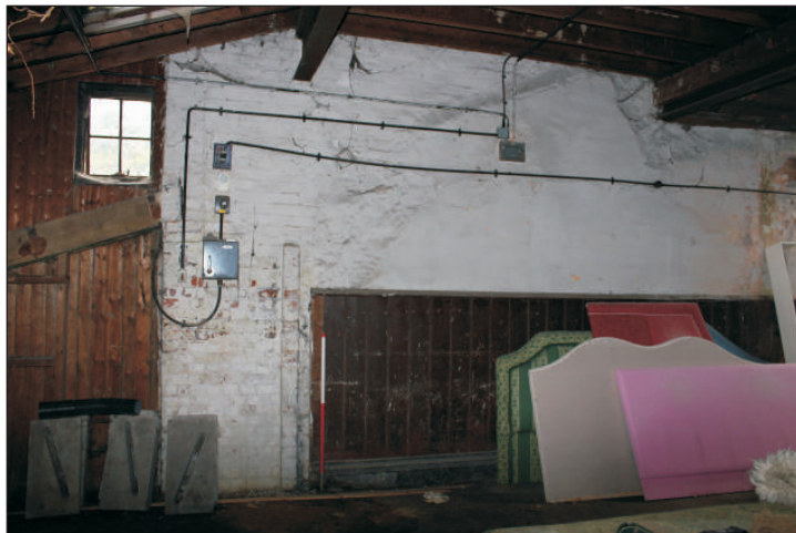
Plate 7: Room 5, east elevation showing panelling with scar of former roofline above, viewed from the east. 1m scale.
