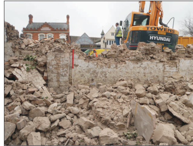
Plate 10: Room 8, the stone piers in the south elevation during demolition, viewed from the north. 1m scale.
