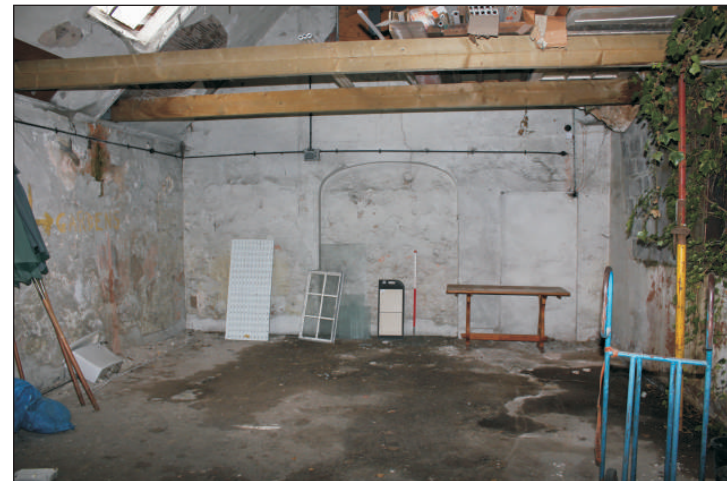
Plate 8: Room 6 showing east elevation with openings, viewed from the west, 1m scale.
