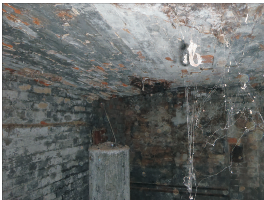
Plate 14: The cellar showing the features in the east elevation, viewed from the west.
