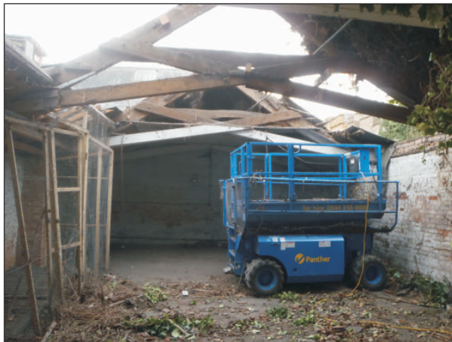
Plate 11: Room 8, the roof as exposed during the demolition, viewed from the east.
