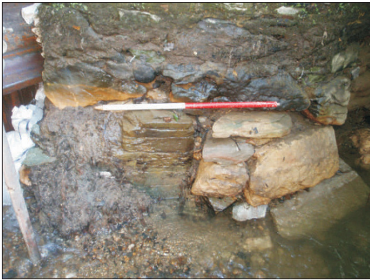
Plate 3: The foundation of the counterfort attached to the central pier, viewed from the south. 1m scale
