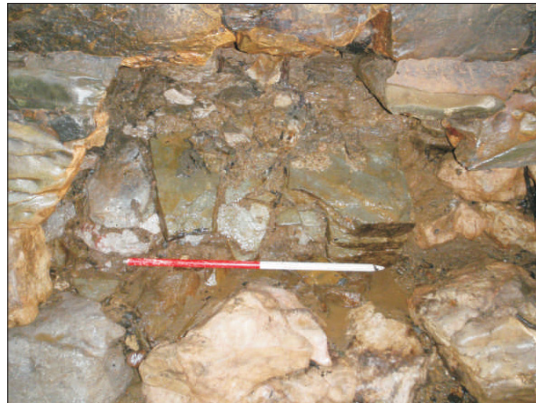
Plate 5: The possible early wall in the south elevation of the central pier, viewed from the south. 1m scale
