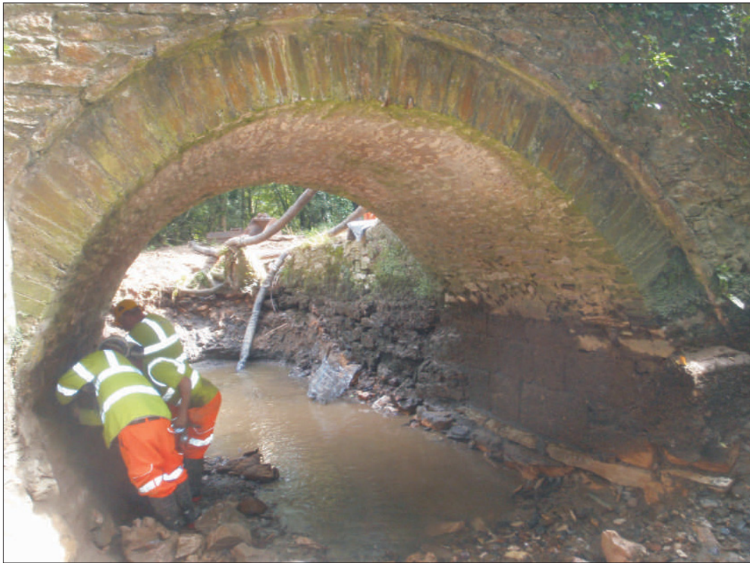
Plate 1: The southern arch showing the south elevation as well as the masonry of the southern abutment, viewed from the northwest
