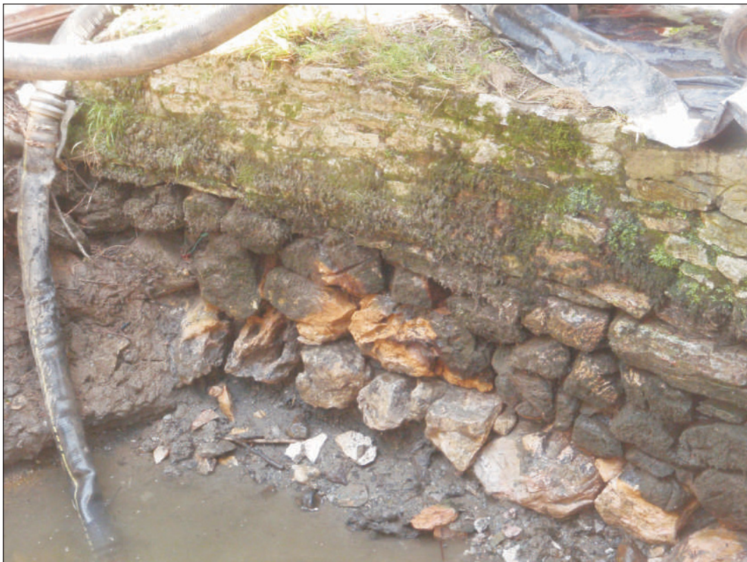
Plate 2: The wing wall east of the southern abutment, viewed from the northwest
