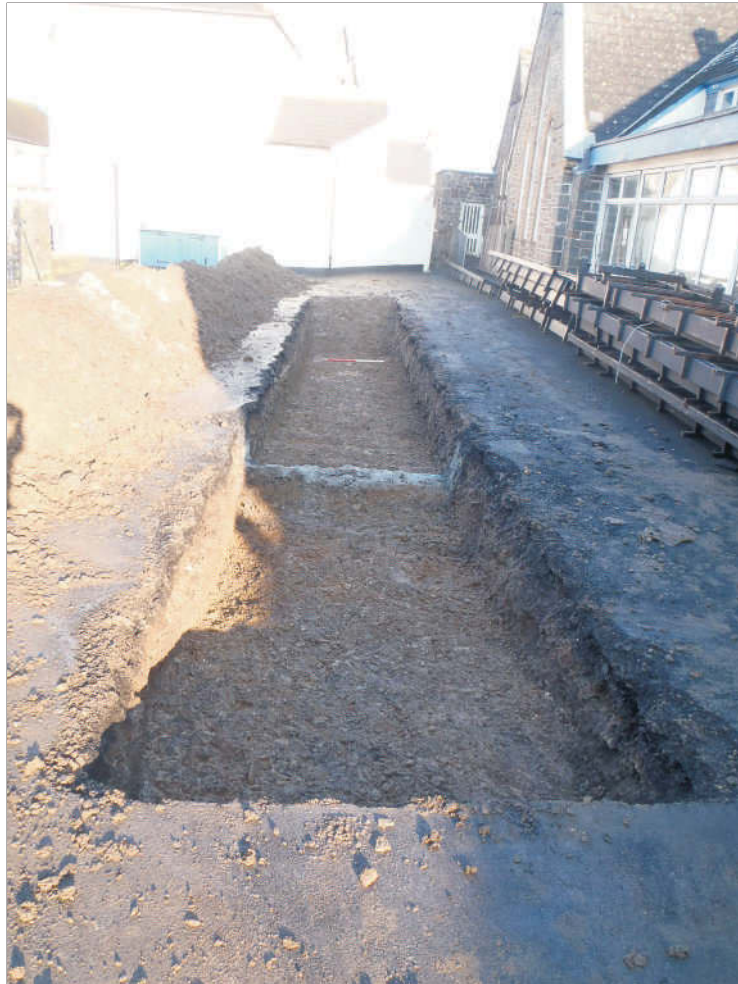
Plate 7: Trench 3, general view (modern service in centre). View from south (scale 1m)
