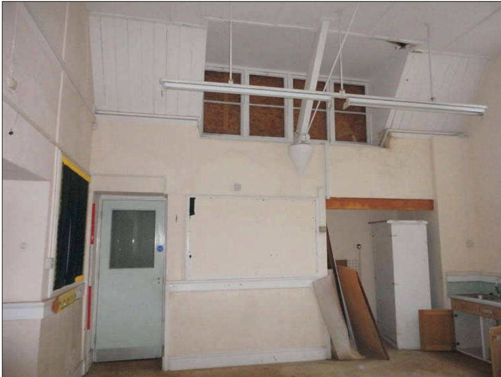
Plate 14: South wall of Infant's schoolroom showing shadow of blocked lancets. 2m scale
