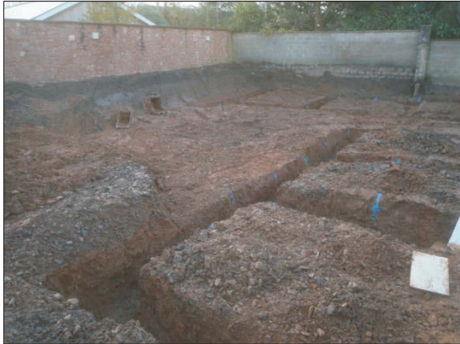
Plate 1: General view of the site after ground reduction and excavation of foundation trenches, viewed from the northeast.
