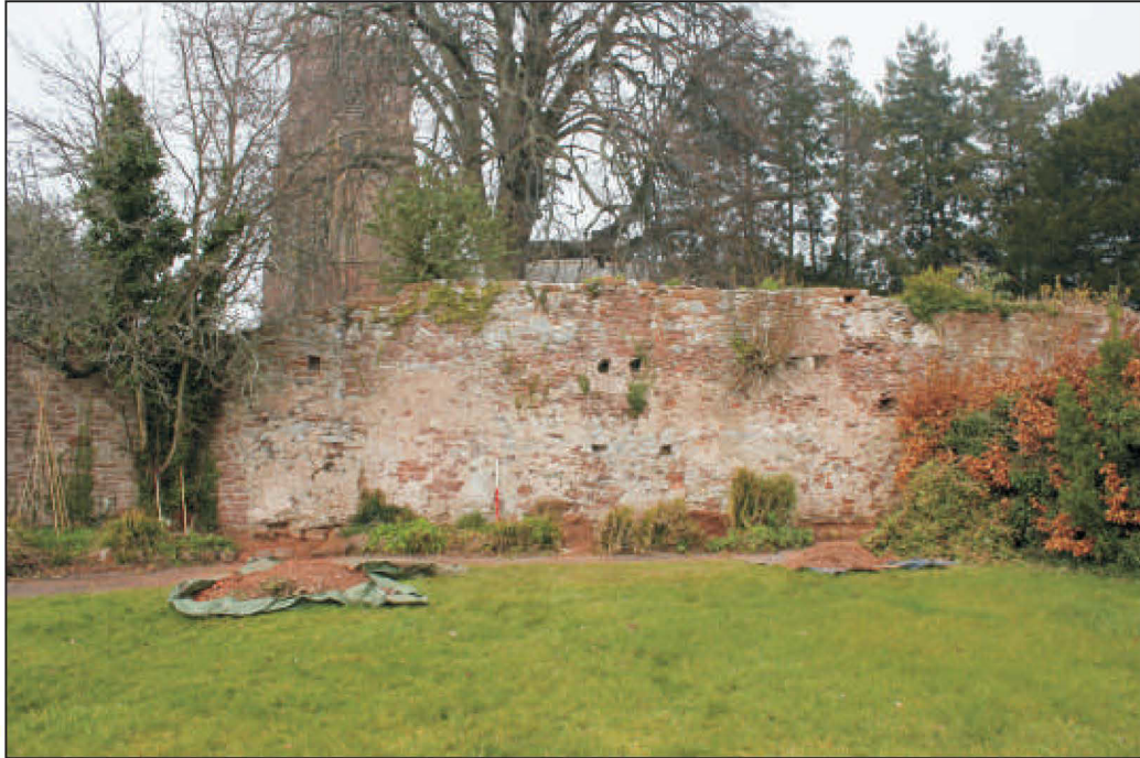
Plate 1: North curtain wall showing F600 with F303 above, viewed from the south. 1m scale.
