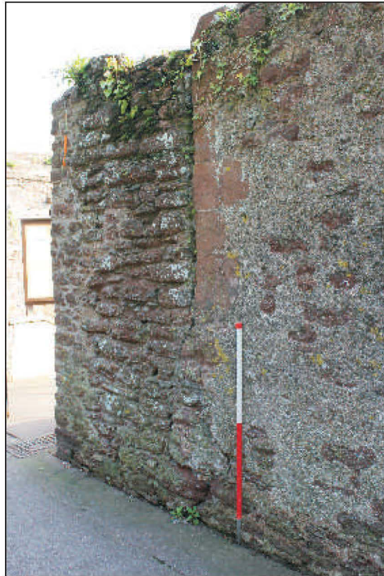
Plate 5: North curtain wall, external elevation showing sandstone jambs of window opening in F303, with later wall F605 beyond, viewed from the northwest. 1m scale.
