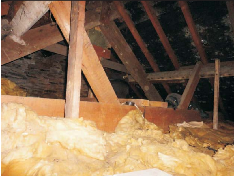
Plate 14: View within the roof, looking west, showing one of the primary trusses
