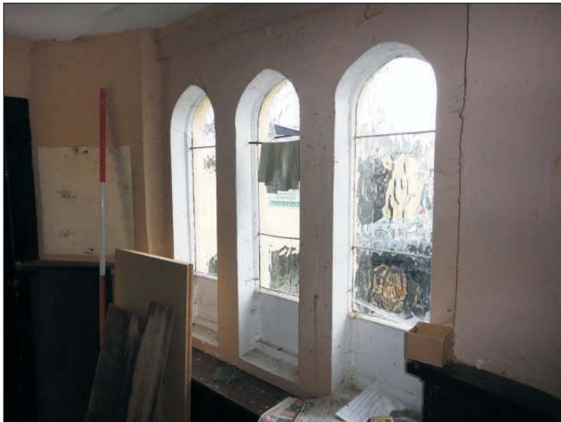
Plate 3: Detail of the window from the interior showing the thick, square mullions and the absence of rebates for shutters. 2m scale
