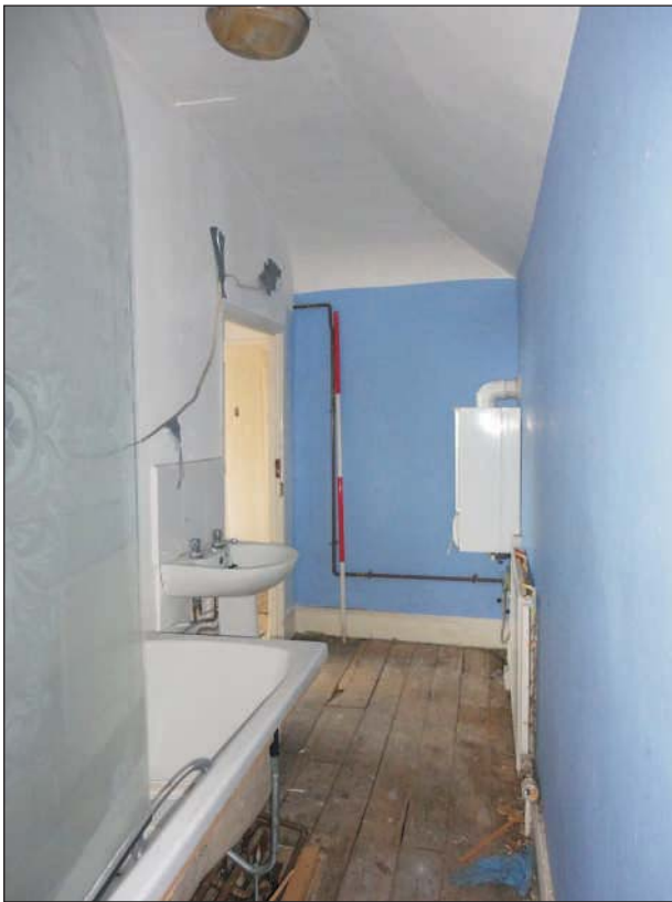
Plate 12: The alcove off the main function room, looking east, showing the domed ceiling and arched opening to the room, infilled by a modern partition. 2m scale
