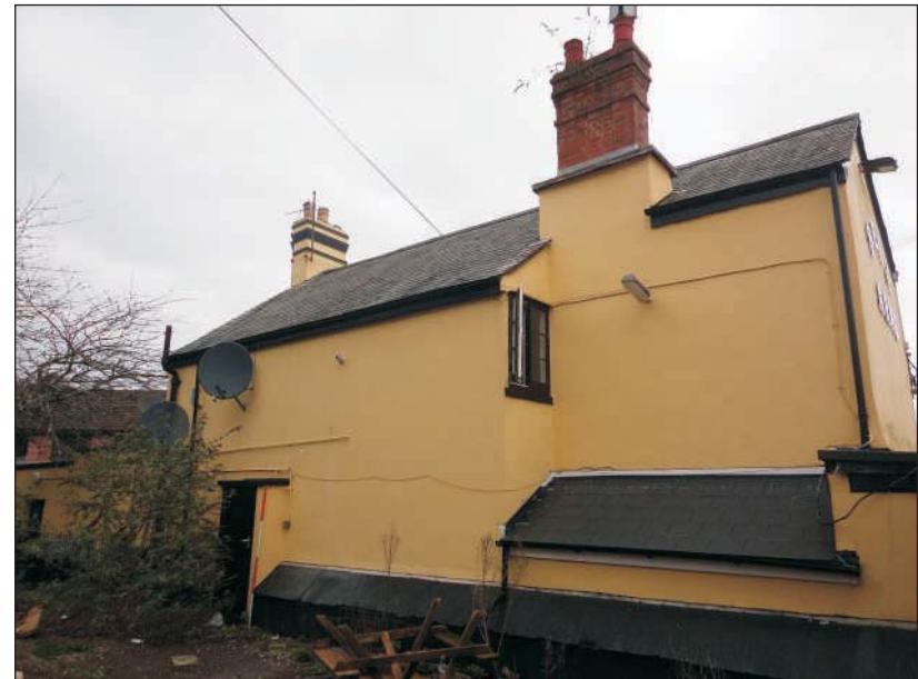
Plate 4: View of the rear elevation showing the presumed French drain running along the base of the wall. 2m scale
