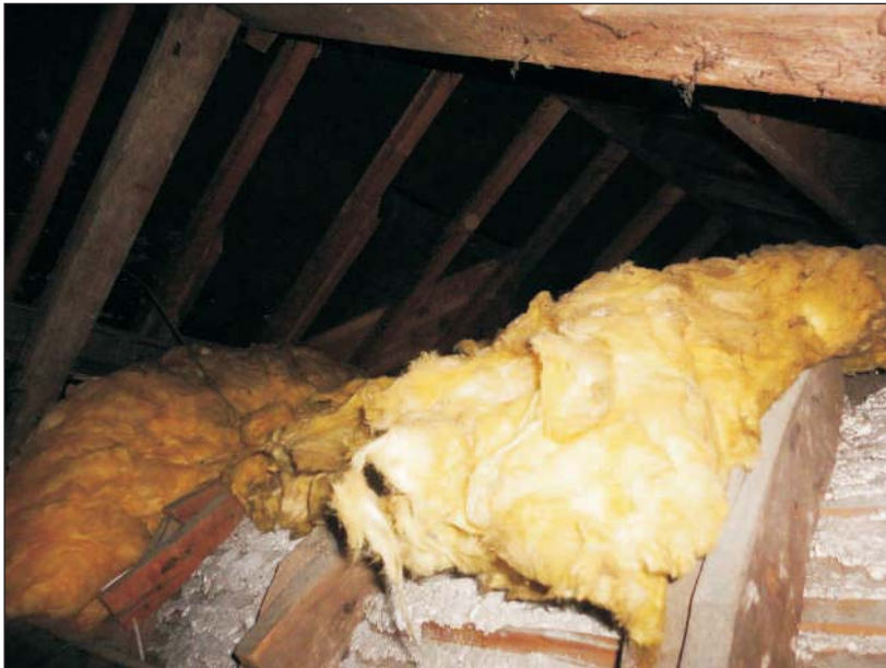
Plate 15: View within the roof, looking east, showing the domed structure over the central bay rising within the roof space
