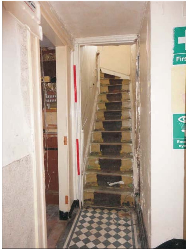
Plate 11: View of the corridor and staircase to the upstairs function rooms. 2m scale
