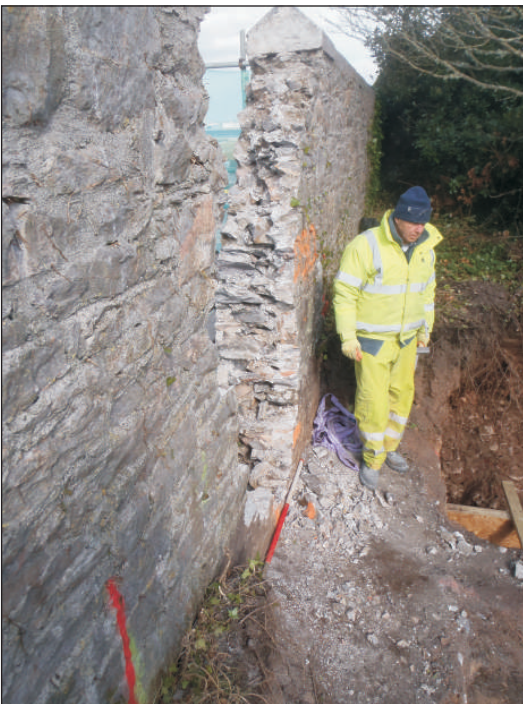
Plate 5: The parapet of the yard boundary wall during breaching, viewed from the southwest. 1m scale.
