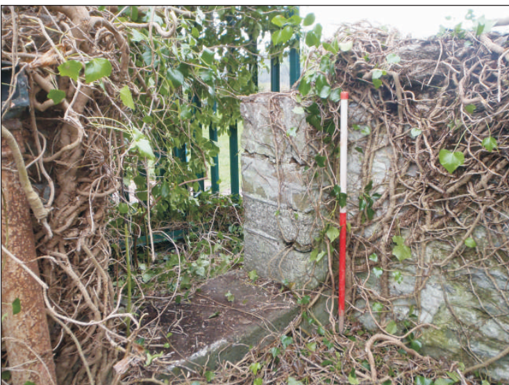
Plate 6: The doorway in the southwest corner of wall 1, viewed from the northeast. 1m scale.
