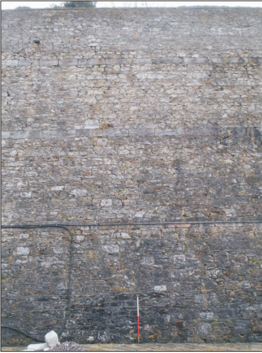
Plate 4: The interior elevation of the yard boundary wall, viewed from the north. 1m scale.
