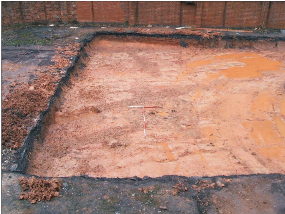
Plate 6: The Car Park, pre-excavation view of the northwestern end showing working conditions and linear post-trenches. 1m and 2m scales.
