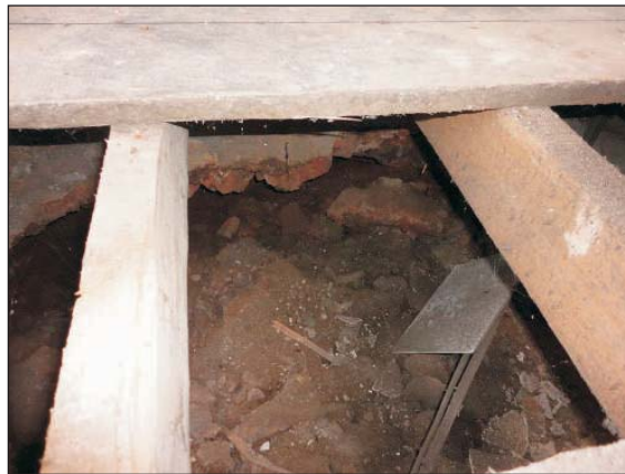
Plate 23: View of the collapsed vault underlying the southeastern ground-floor room of Acacia House.
