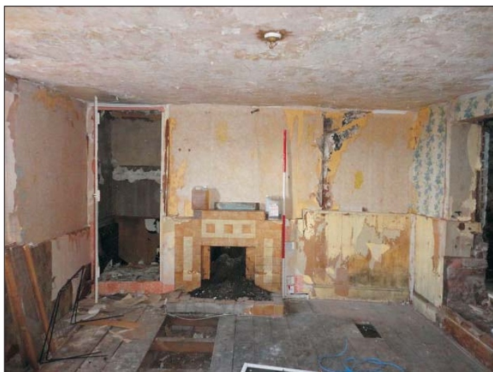
Plate 11: View of the northwestern wall of the main room in the service wing after stripping out. Scale 2m
