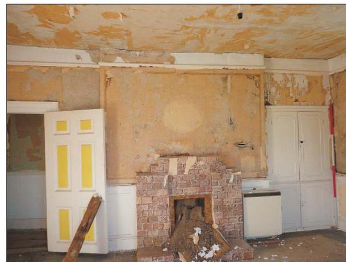
Plate 10: View of the northeastern wall of the main bedroom showing features after stripping out. Scale 2m
