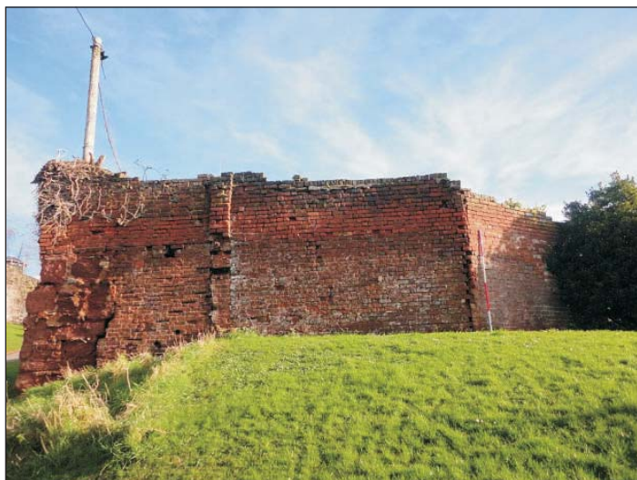
Plate 3: Detail of the corner of the site boundary showing successive brick builds, evidence of a staircase and the baulk of early masonry at the corner.
