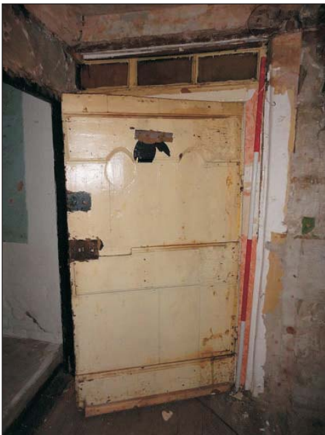
Plate 7: Detail of the historic door to the service wing showing original 'L'-hinges. Scale 2m
