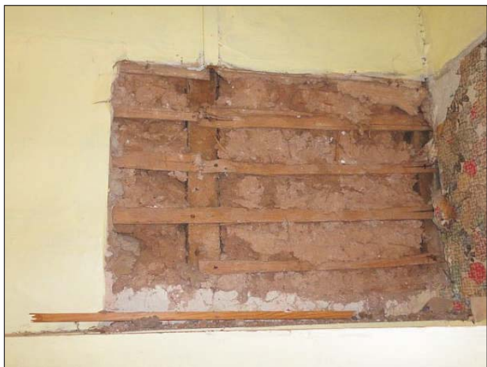
Plate 15: Detail of the method of construction, utilising cob infill panels, on the first floor of the service wing.
