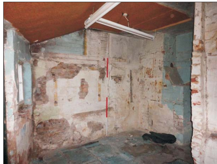
Plate 14: View of the lean to after stripping out showing the fireplace and chimney in the southeastern wall. Scale 2m
