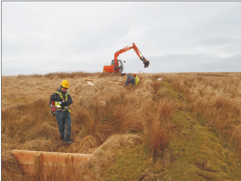
Plate 1: General view of works showing construction of wooden dams, viewed from the east
