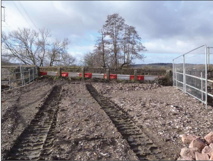
Plate 1: Stoke Canon Bridge, west parapet prior to removal of posts, viewed from the northeast
