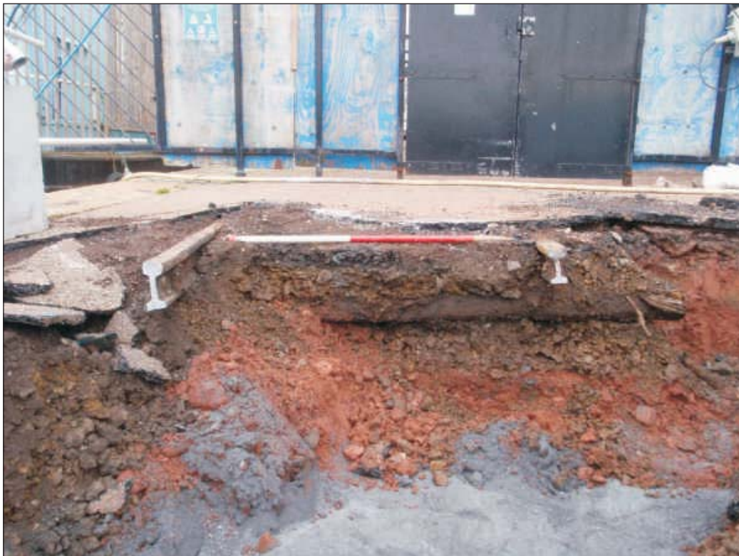
Plate 8: Section through the trench for the siding rails at the north end of the site, viewed from the southeast (scale 1m)
