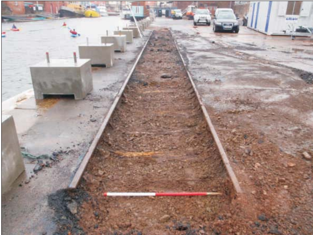
Plate 7: The exposed siding rails at the southern end of the site, viewed from the southeast (scale 1m)
