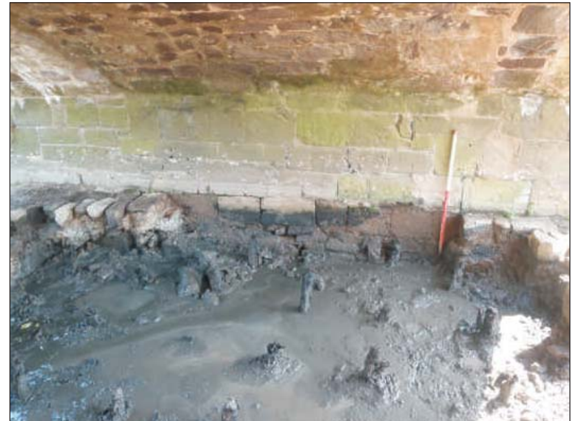
Plate 8: View of part of the bridge abutment exposed once the invert had been removed, also showing stakes 106. Taken from the north. Scale 1m
