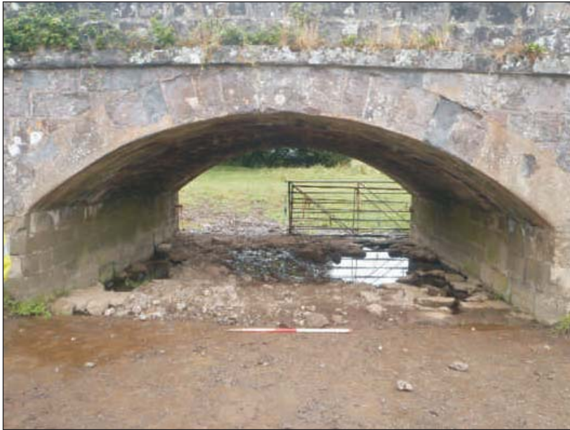
Plate 1: View of the invert before commencement of the repairs, taken from the east. Scale 1m
