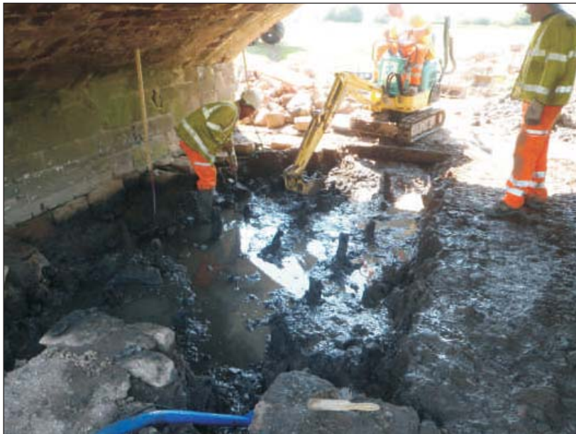
Plate 7: General working shot taken during the excavation of the scour hole showing stakes 106. Taken from the east
