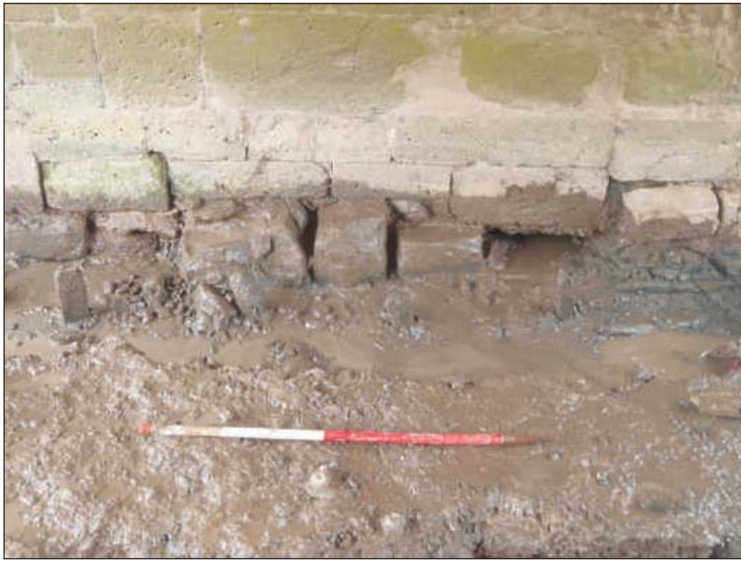
Plate 11: View of part of the bridge foundations (111), taken from the south. Scale 1m
