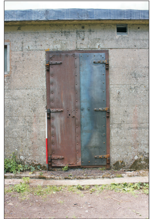
Plate 5: The doors in the eastern elevation showing the evidence for the hood above, viewed from the east. 1m scale.
