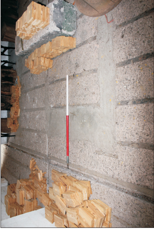
Plate 9: The floor of the receiver room showing the battens for the floor joists and infilled cable ducts, viewed from the east. 1m scale.
