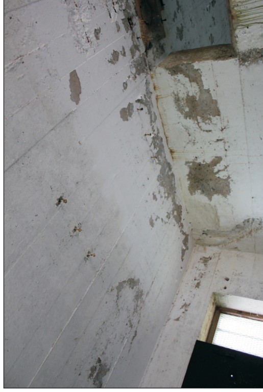
Plate 11: The fixings on the ceiling of the transmitter room for the aerial array turning gear, viewed from the southwest.
