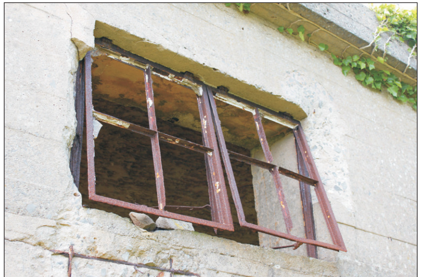
Plate 7: An original window frame at Oxwich Bay, viewed from the southeast. Photo: Andrew Passmore
