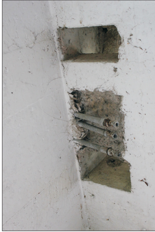
Plate 10: The ducts in the telephone room, viewed from the southwest.
