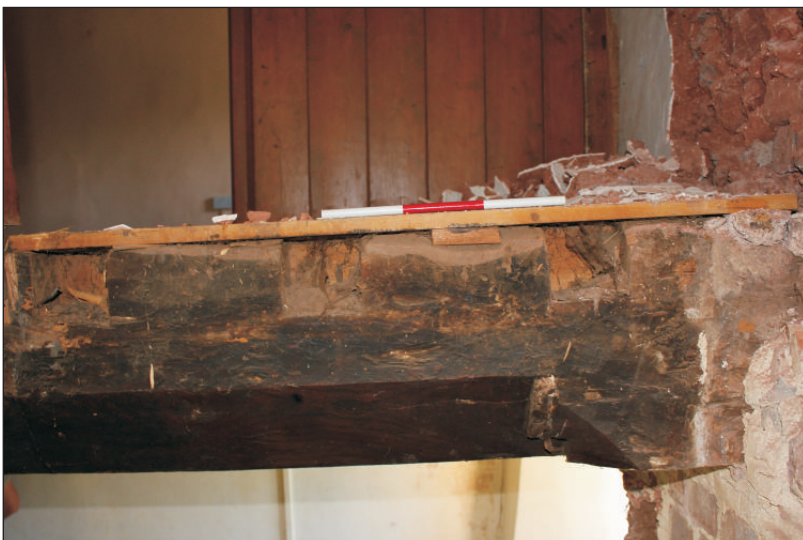
Plate 9: Exposed floor joist sockets in the beam following removal of the stairs, viewed from the northeast. 0.30m scale.
