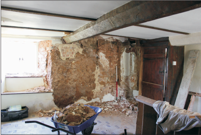
Plate 4: The west wall interior elevation after removal of plaster, viewed from the south. 1m scale.
