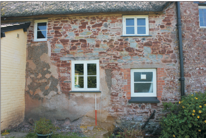
Plate 2: The west wall external elevation prior to removal of render, viewed from the northwest. 1m scale.
