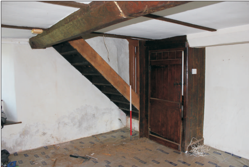
Plate 7: The stairs and adjacent door after removal of the partition, viewed from the south. 1m scale.
