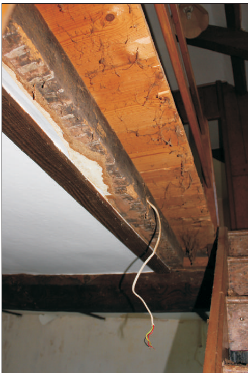
Plate 8: The exposed floor joist, showing evidence of a former ceiling, viewed from the north.
