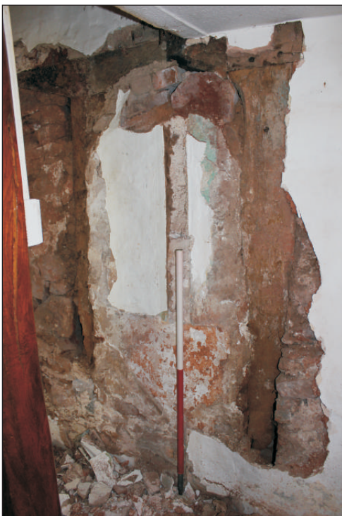
Plate 6: The northern of the two blocked doorways, viewed from the east. 1m scale.
