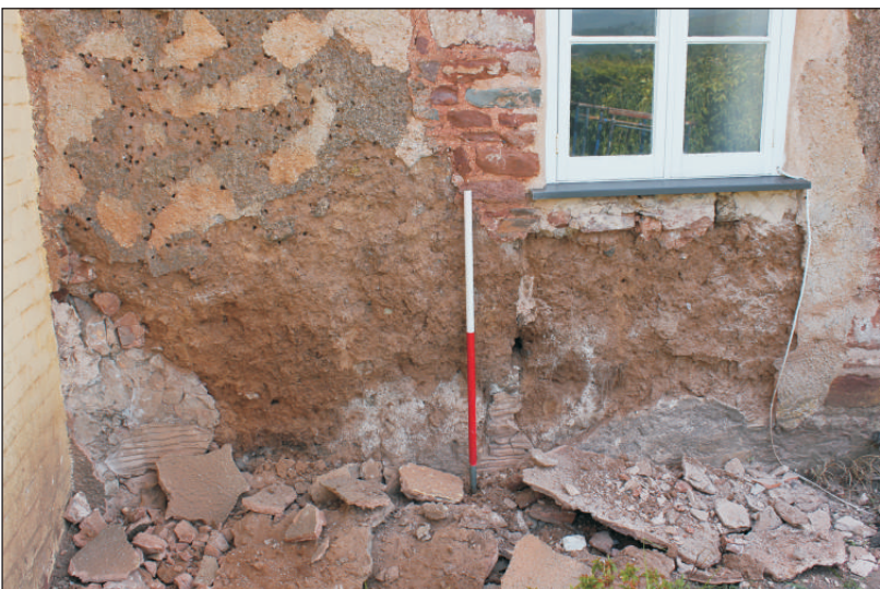
Plate 3: The west wall external elevation after removal of render exposing primary cob fabric, viewed from the northwest. 1m scale.
