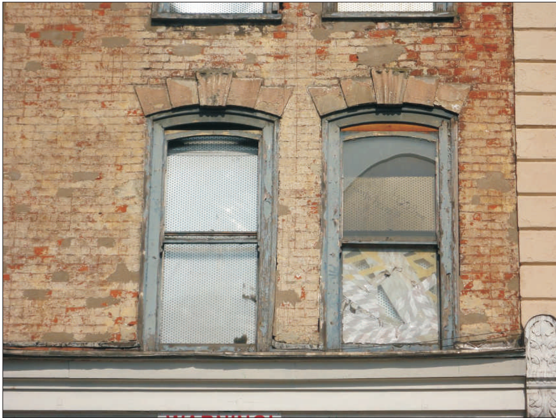
Plate 3: Segmental-headed windows with flush-framed sash boxes typical of the early-mid 18th century in the upper storey of No 37 Stokes Croft
