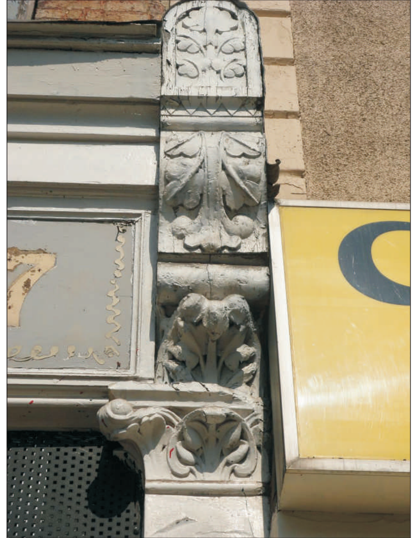
Plate 6: Detail of the ornamental corbel at the north-eastern side of the shop front, showing continental Gothic detail on the capital
