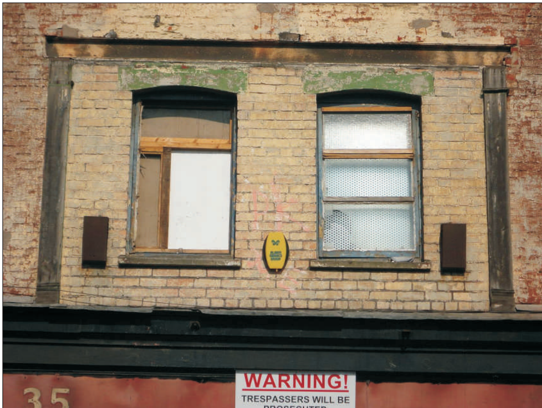
Plate 4: The remains of a late 19th-century first-floor display window at No. 35, blocked in the 20th century
