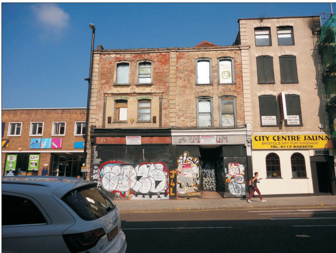
Plate 2: Details of the façades of the houses showing the offset windows in Nos 37 and 39 and typical architectural details
