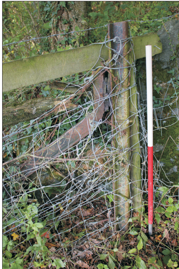
Plate 8: A fence post of reused rails on the northwest side of the bridge, viewed from the south. 1m scale.
