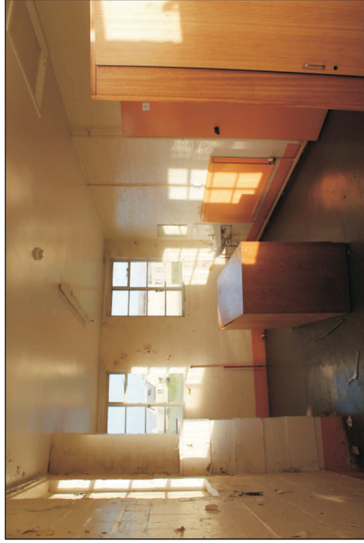
Plate 15: Building 3, accommodation block, interior showing chimney stack, viewed from the east. 1m scale
