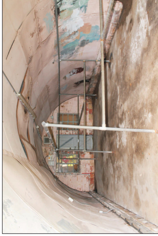
Plate 16: Building 64, interior of a curved asbestos hut, viewed from the west. 1m scale
