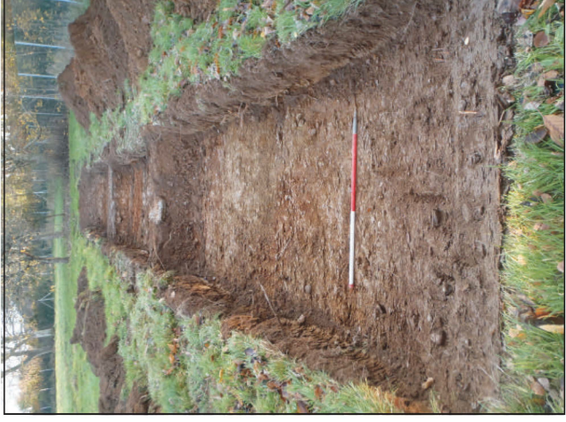
Plate 6: Trench 28 viewed from the west showing footings of demolished buildings. 1m scale
