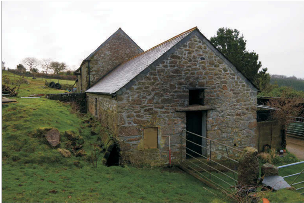
Plate 3: Room A, west elevation, also showing collapsed retaining wall on north side of building, viewed from the northwest. 1m scale.
