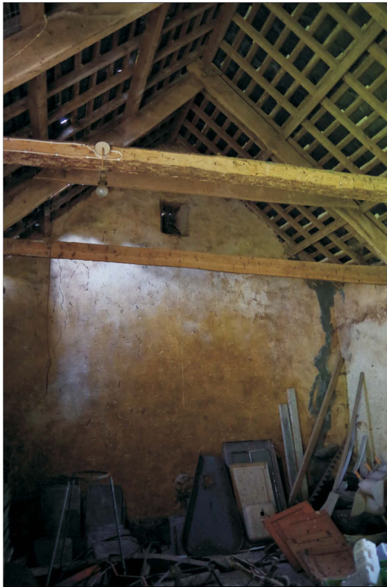
Plate 7: The first floor of room B showing the roof structure, viewed from the southeast.
