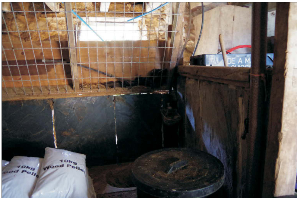
Plate 6: The interior of room B showing the slate stalls, viewed from the south.
