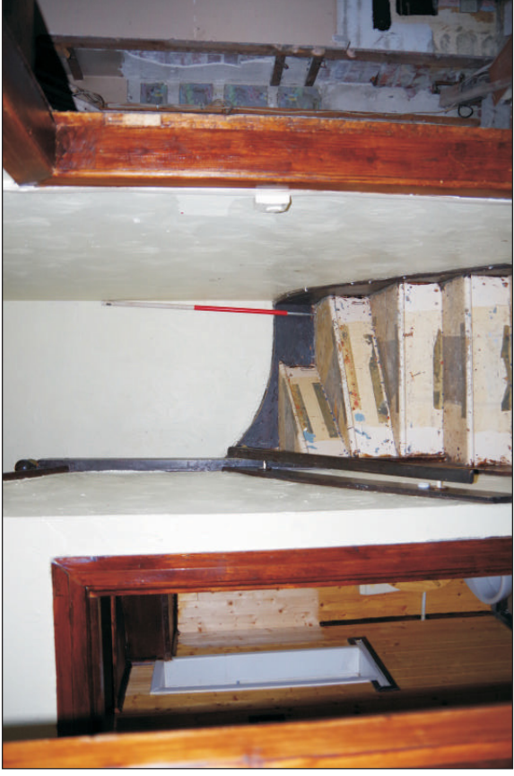
Plate 6: No. 23 Ash Grove, the hall and stairs, viewed from the east. 1m scale.
