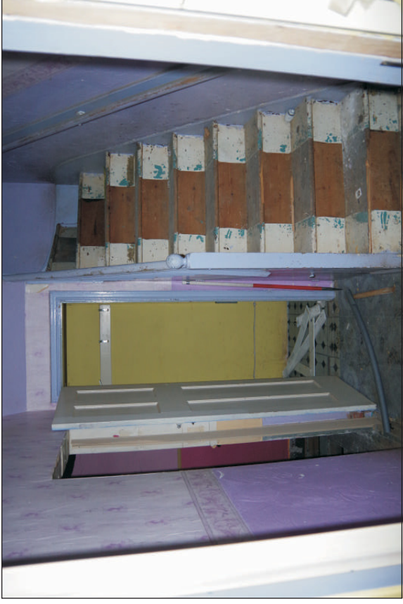
Plate 2: No. 5 Ash Grove the hall showing stairs and a typical original door, viewed from the southeast. 1m scale.
