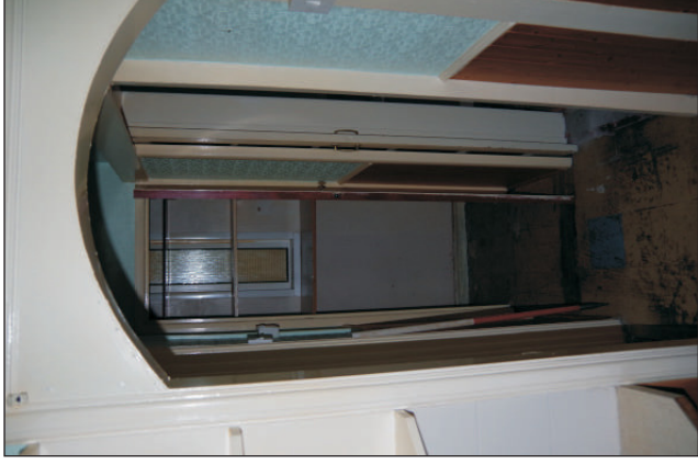
Plate 8: No. 38 Ash Grove, the ground-floor corridor showing the arched opening from the kitchen, viewed from the west. 1m scale.
