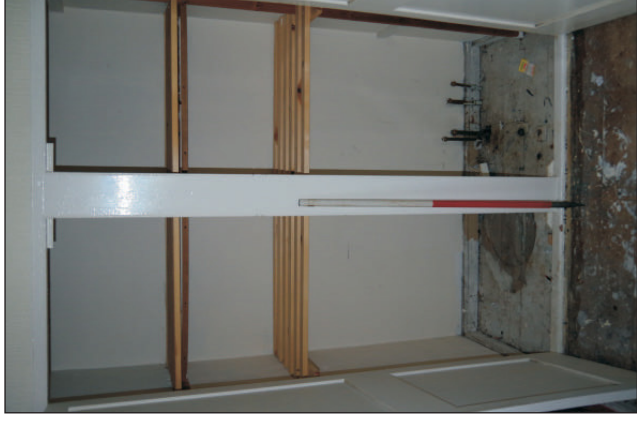
Plate 4: No. 11 Ash Grove, the airing cupboard in the master bedroom, viewed from the southeast. 1m scale.
