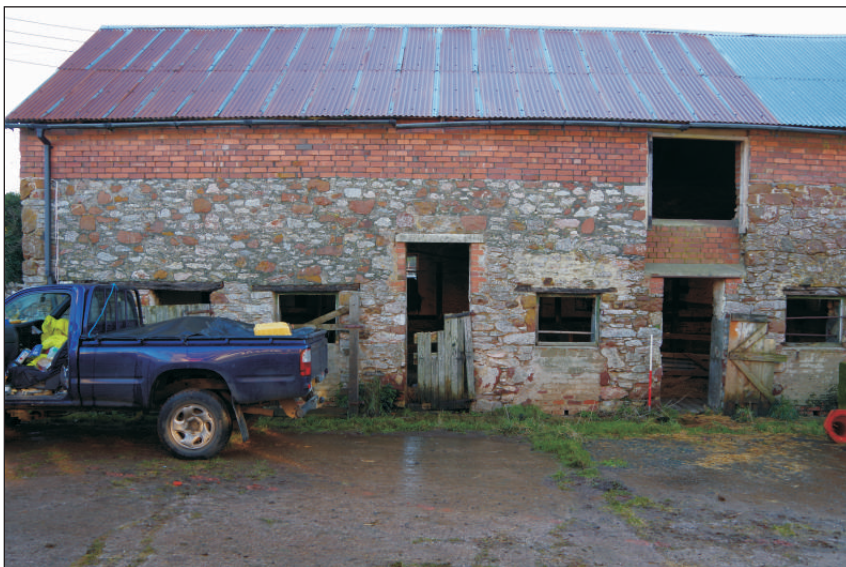
Plate 2: Building 1, southwest elevation, north end, showing raised rooflines and altered openings, viewed from the southwest. 1m scale.
