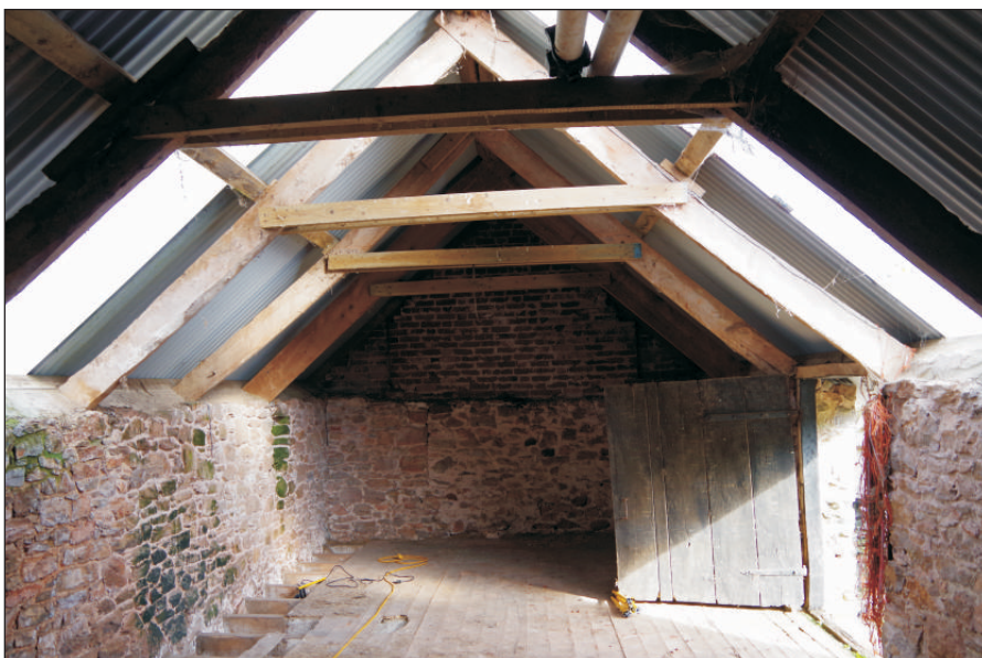
Plate 12: Building 4, first floor showing roof timbers and break in northeast elevation, viewed from the southeast
