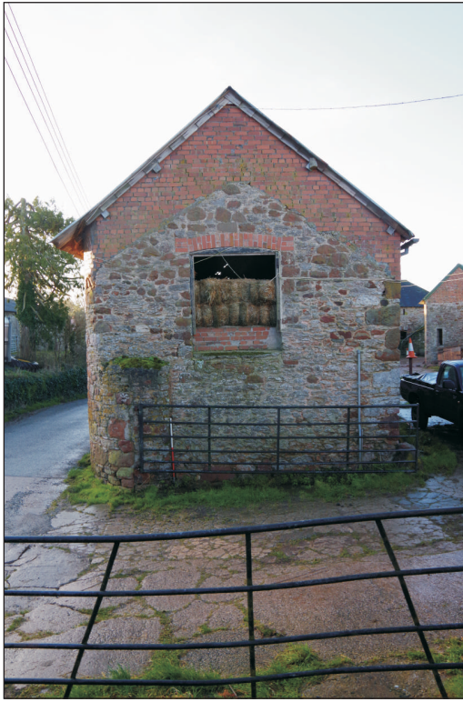
Plate 1: Building 1, northwest elevation showing raised rooflines, viewed from the northeast. 1m scale.
