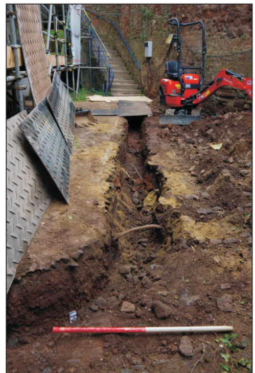
Plate 16: View of the east yard service trench, view from the south (scale 1m)
