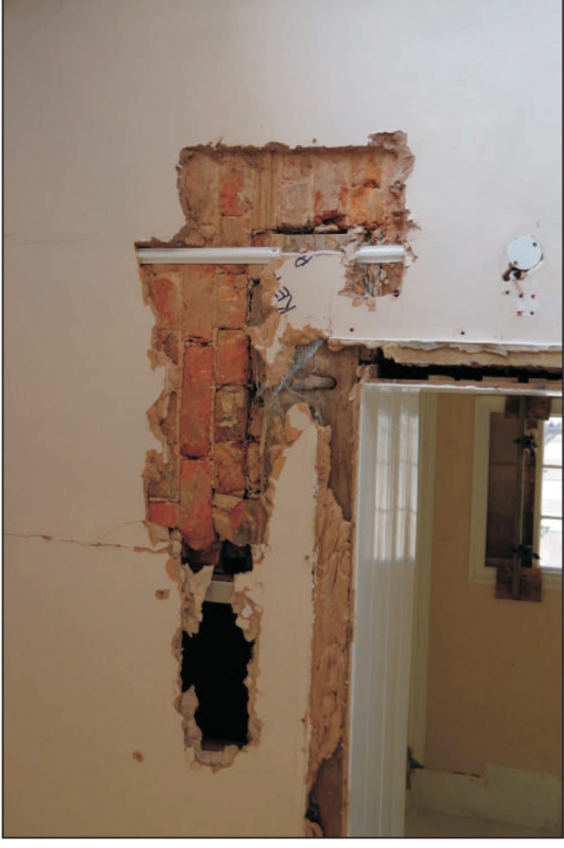
Plate 10: First floor, east wall of Room F5, primary building brickwork (scale 1m)
