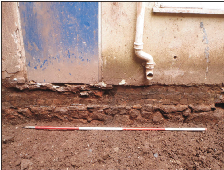
Plate 13: South wall foundations F108 and F109, view from the south (scale 2m)
