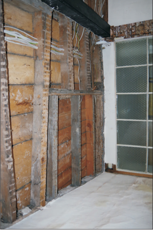
Plate 6: The joist arrangement showing the location of the former stairs, viewed from the north.
