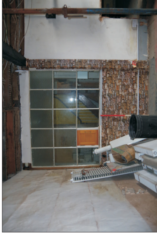
Plate 4: The partition between the shop and the kitchen, viewed from the north. 1m scale.
