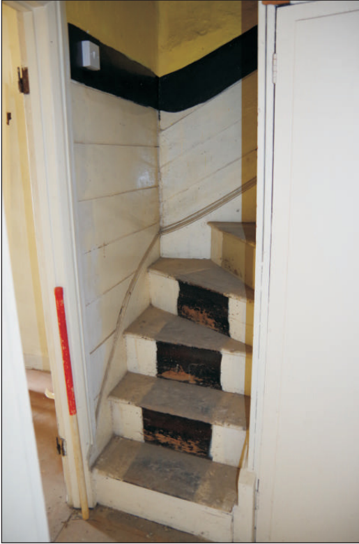
Plate 9: The stairs to the second floor, viewed from the southwest. 1m scale.
