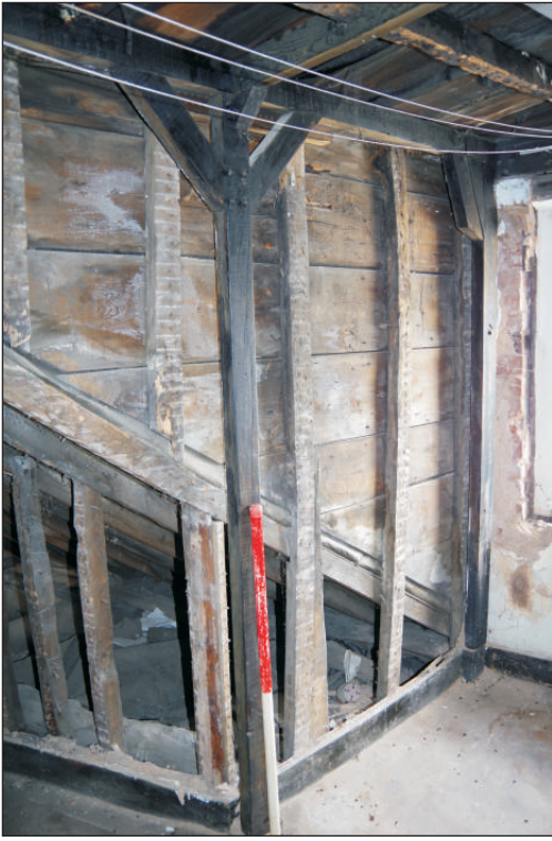
Plate 12: The second floor stairwell showing secondary timbers, viewed from the southwest. 1m scale.
