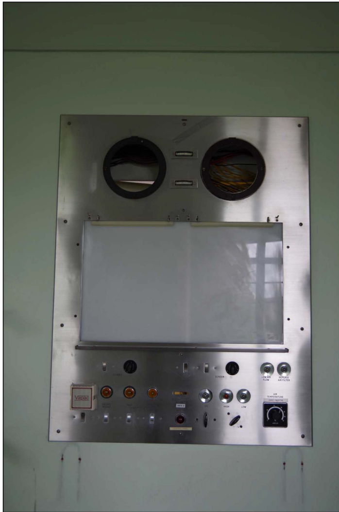
Plate 18: The X-ray light box and control panel in the operating theatre, looking southeast
