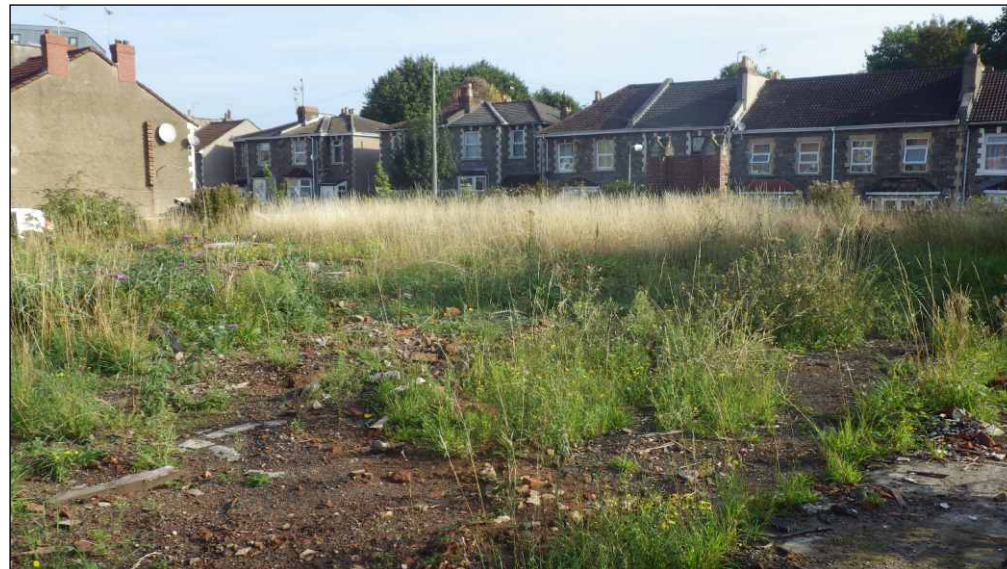
Plate 2: General site view, area of demolished Granby House, view to the north-east
