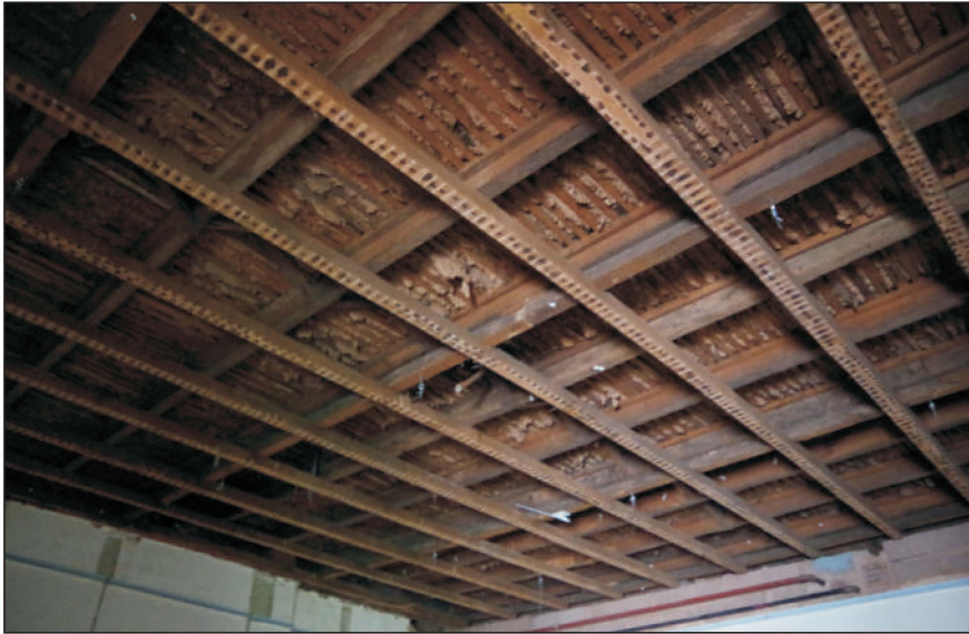
Plate 5: The pugging in the ceiling of the speech therapy room, viewed from the west
