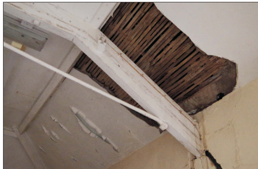
Plate 2: Lath and plaster ceiling covering in the first floor east room of the central range, viewed from the southeast
