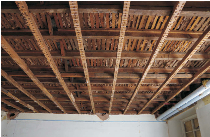
Plate 7: The pugging in the ceiling of the chiropody room, viewed from the west
