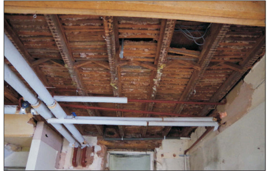
Plate 6: The pugging in the ceiling of the waiting room, viewed from the southwest
