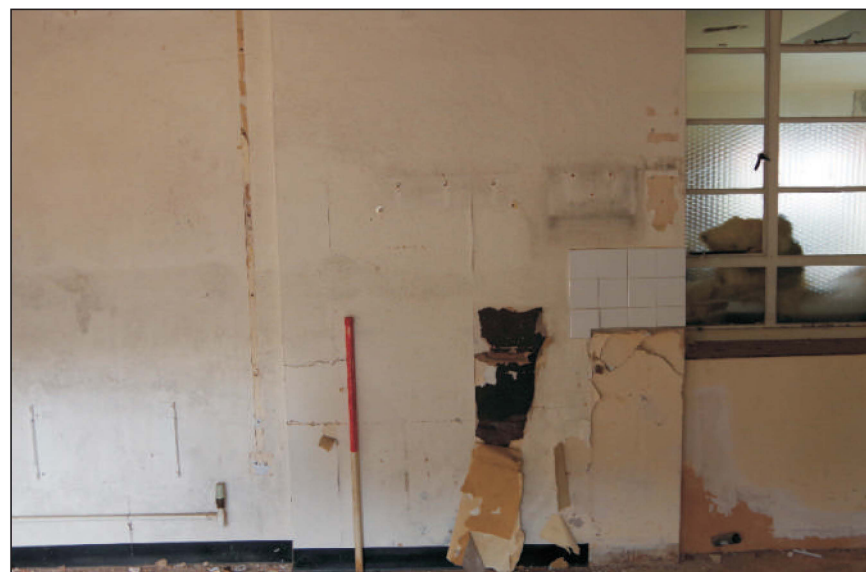
Plate 4: The blocked fireplace in the chiropody room of the central range, viewed from the south. 1m scale
