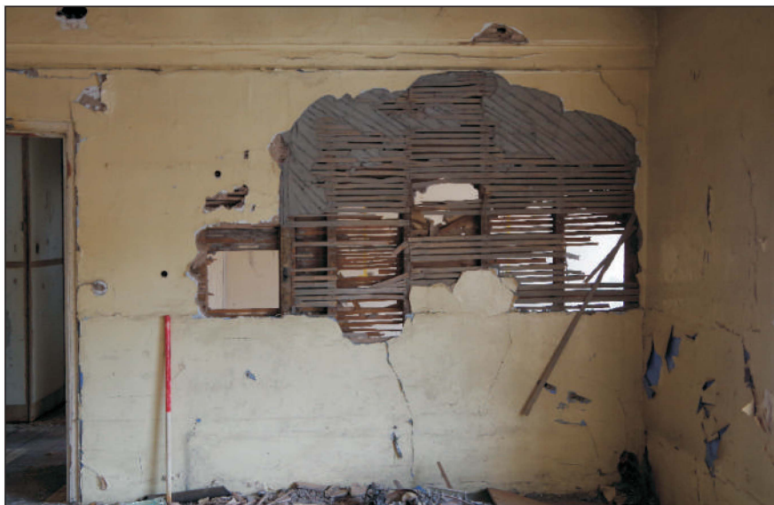
Plate 1: Lath and plaster wall covering in the west room of the central range, viewed from the west. 1m scale
