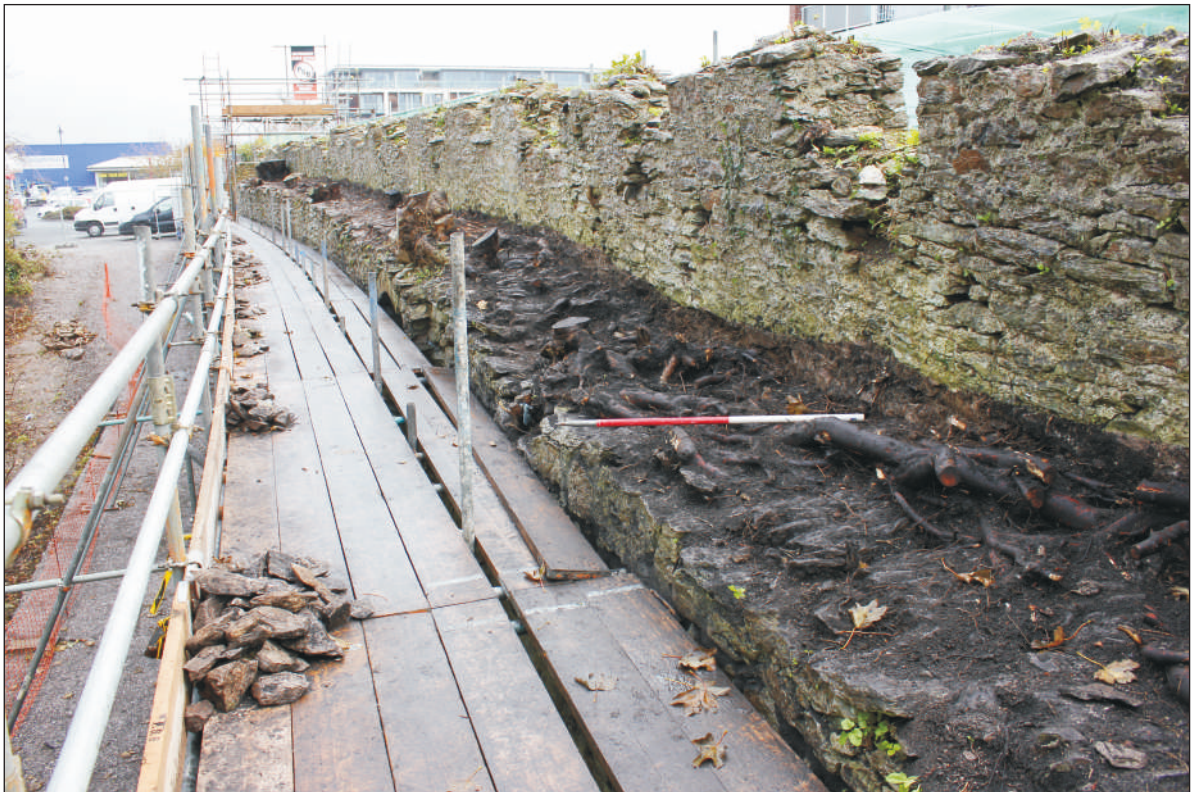
Plate 8: Tree root damage at the east end of the wall walk, looking east. 1m scale.
