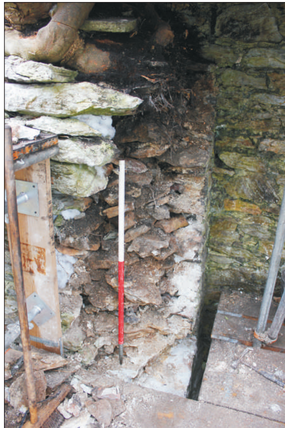
Plate 10: General view during repairs to the west end of the wall walk, looking south. 1m scale.
