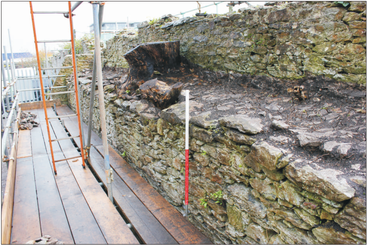
Plate 9: Tree root damage at the east end of the wall walk, looking east. 1m scale.
