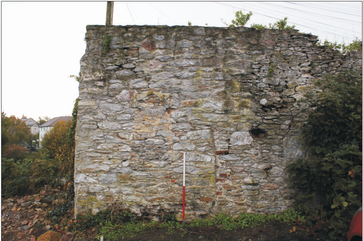
Plate 11: The north elevation at the east end of the wall, looking south. 1m scale.
