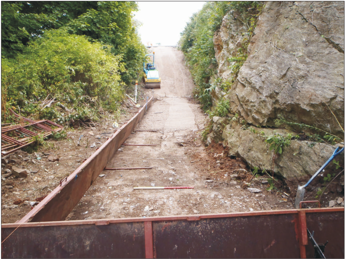
Plate 1: General view of groundworks for the earth bank, looking east. 1m scale.
