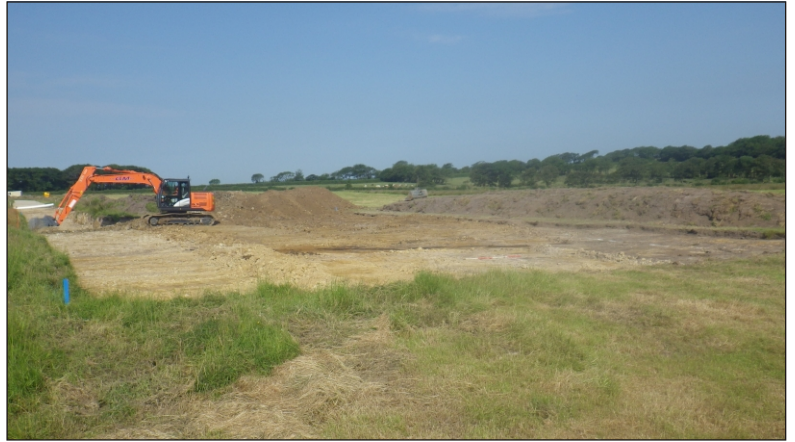
Plate 5: Stripping of the crane pad looking northwest with F016 visible as the black line behind the scale.
