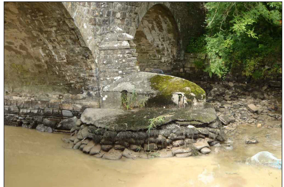
Plate 4: Pier 2 showing 20th-century repairs to the cutwater, viewed from the northeast
