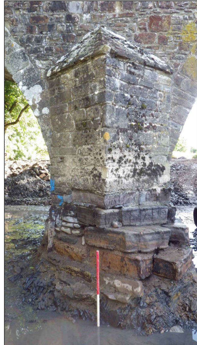
Plate 6: The downstream cutwater on pier 2 showing the construction details of the masonry abutting the pier, viewed from the southwest. Scale 1m
