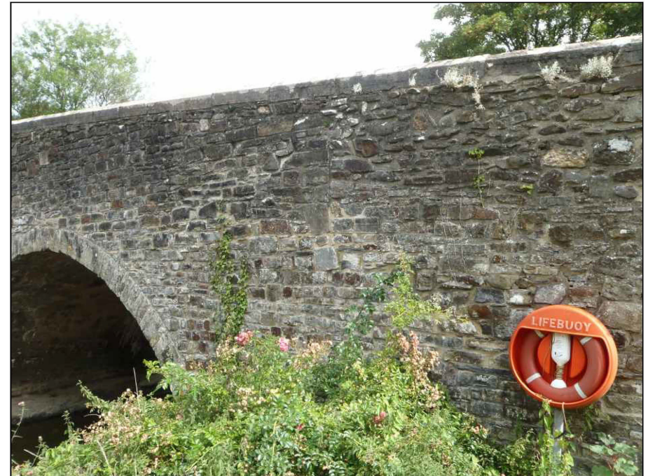
Plate 16: The vertical break in the southern parapet, viewed from the south
