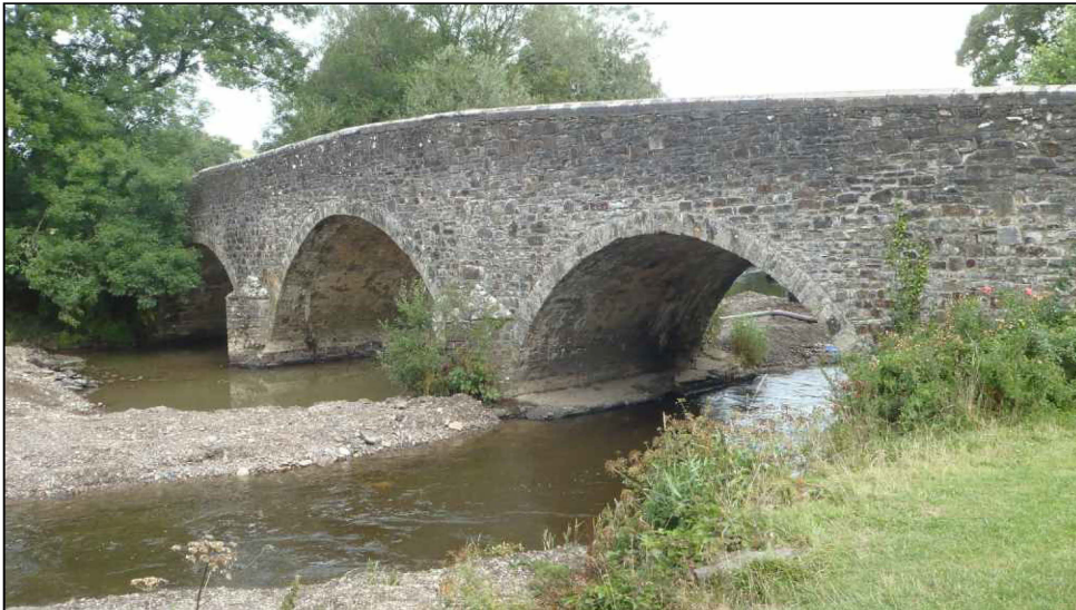
Plate 1: View of the downstream elevation of the bridge prior to commencement of groundworks, viewed from the southeast
