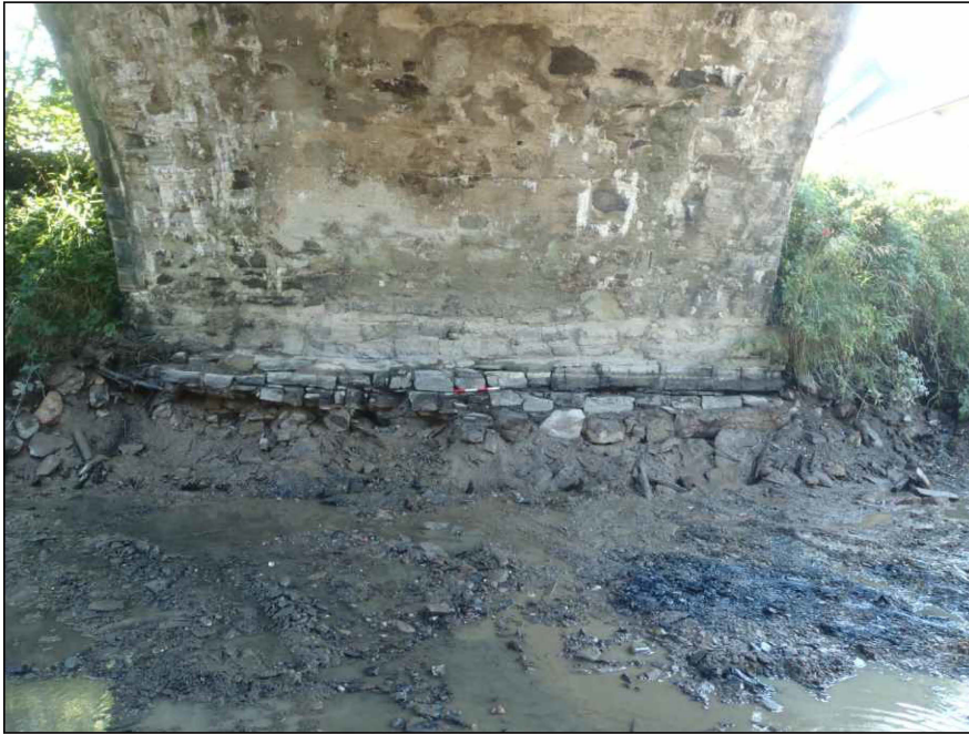
Plate 8: The foundations of pier 3 showing stakes 105, viewed from the northwest. Scale 0.40m
