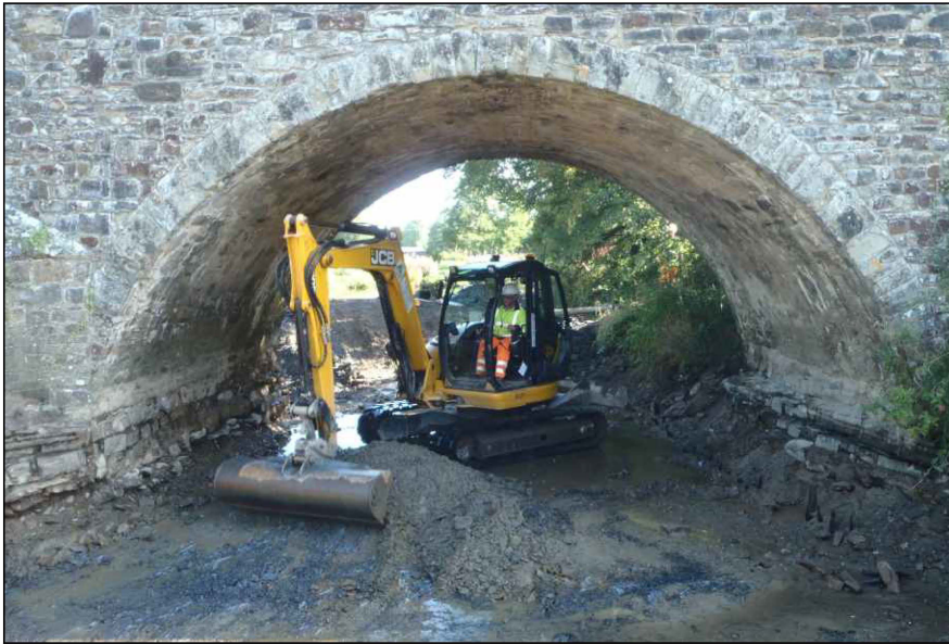
Plate 5: View of excavations between pier 1 and 3 showing the elevation of the arch, viewed from the southwest
