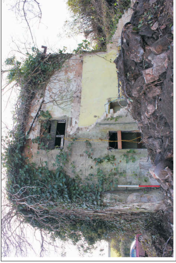
Plate 3 : The north elevation following partial demolition of the kitchen extension, viewed from the northwest. 1m scale
