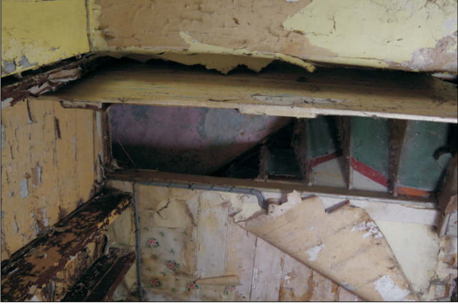
Plate 9: The stairs in the rear room, viewed from the east looking in the rear door
