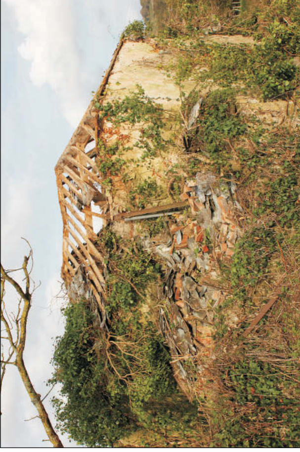
Plate 10: The southwest side of the roof during demolition showing exposed timbers, viewed from the southwest
