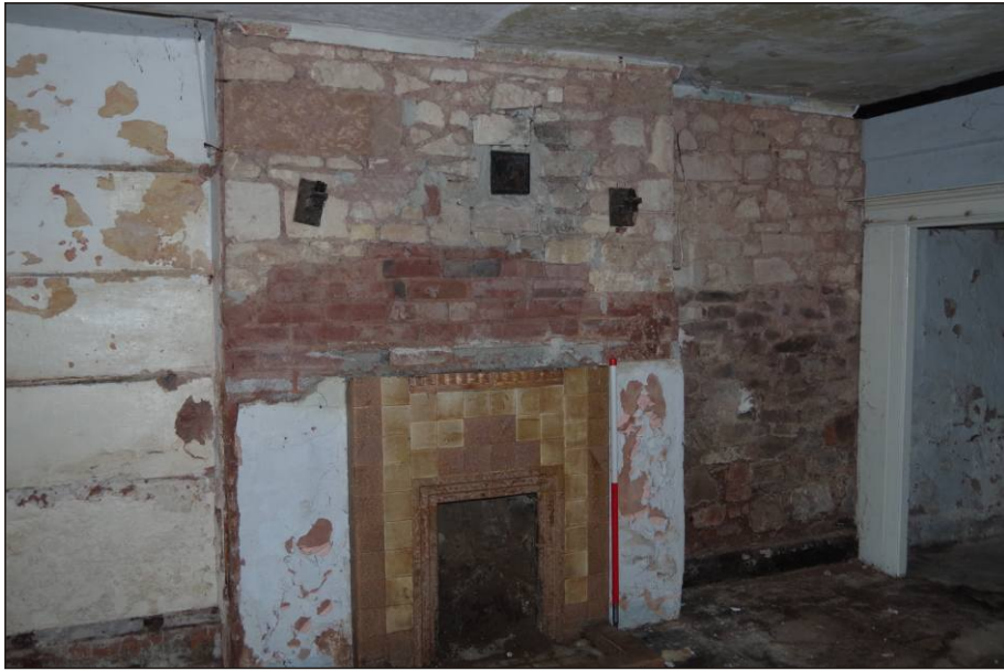
Plate 26: Room LGF6 showing horizontal break in main wall, looking northeast. 1m scale
