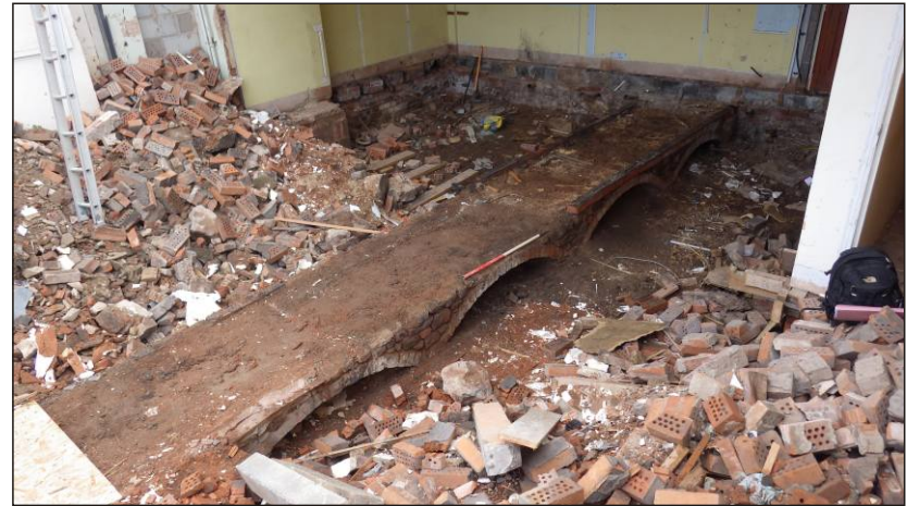
Plate 6: Nos 1 and 2 St Andrew Street, top of cellar arches looking northeast. 1m scale
