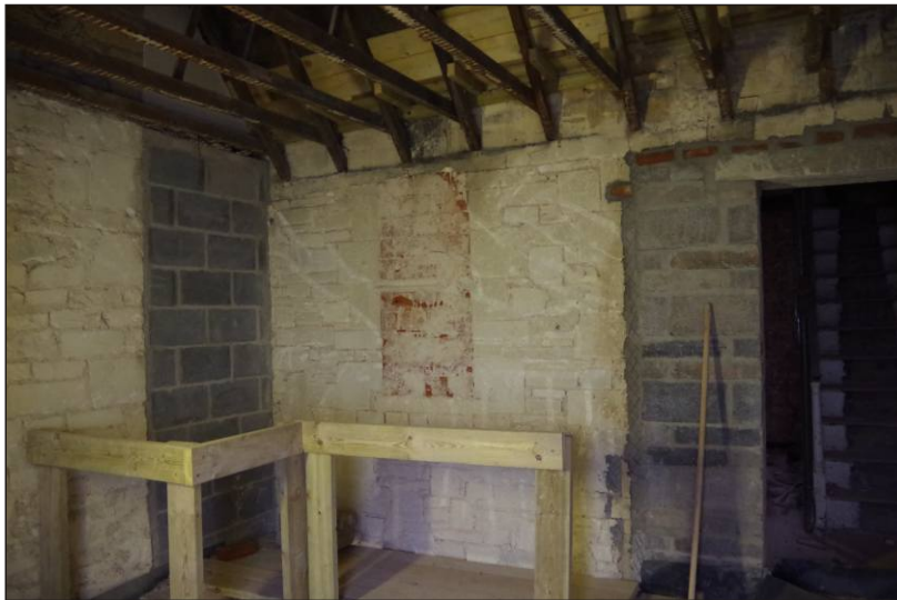
Plate 24: Room FF1 in No. 10 – blocked cupboards as well openings in west elevation, looking southwest
