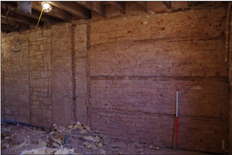
Plate 20: Room GF3 – rebuild west end of south elevation, looking southeast. 1m scale
