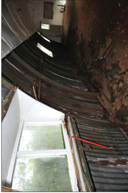
Plate 5: The hall during demolition showing the ribs and purlins supporting the outer covering and inner lining, viewed from the east.
