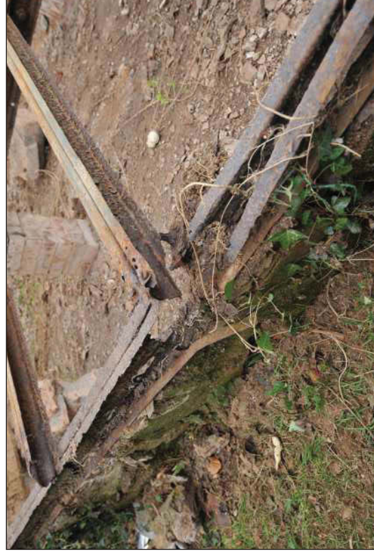
Plate 4: A close-up view of the metal frame base, viewed from the northwest.
