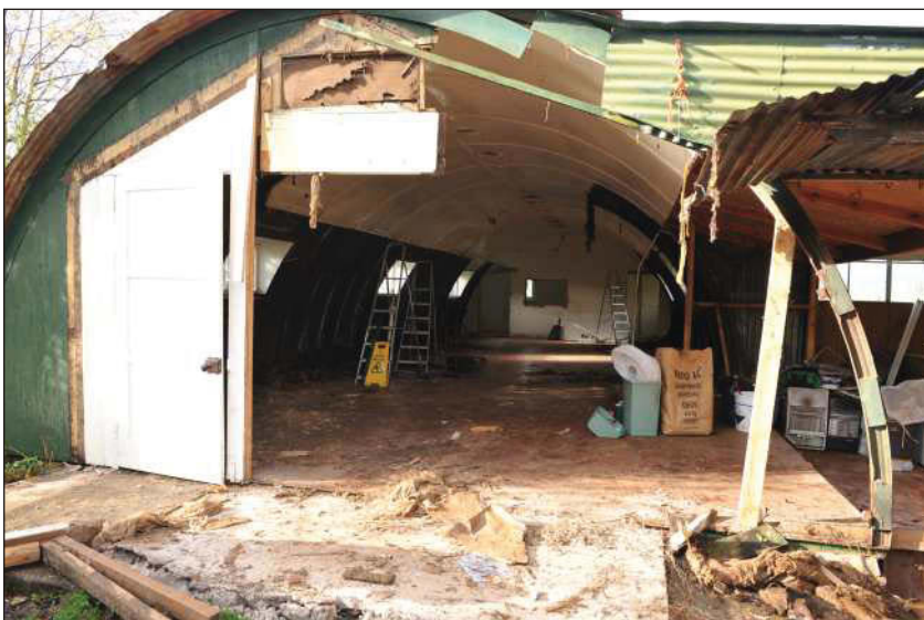
Plate 11: The hall during demolition following removal of the lobby, viewed from the east.
