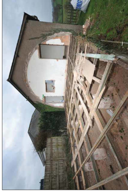
Plate 3: The hall during demolition showing the metal frame base supported on brick piers, and the internal wall to the kitchen, viewed from the east.
