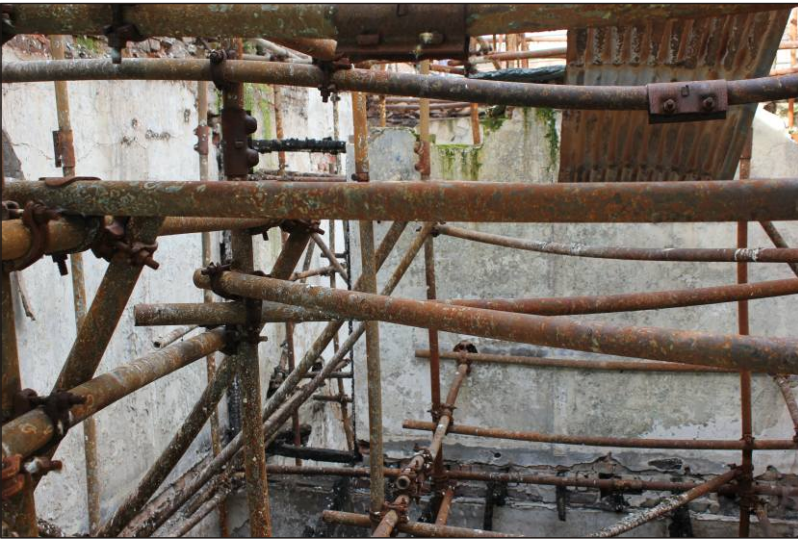
Plate 14: The second-floor partition wall showing the scar of the removed/destroyed partition, viewed from the southeast.
