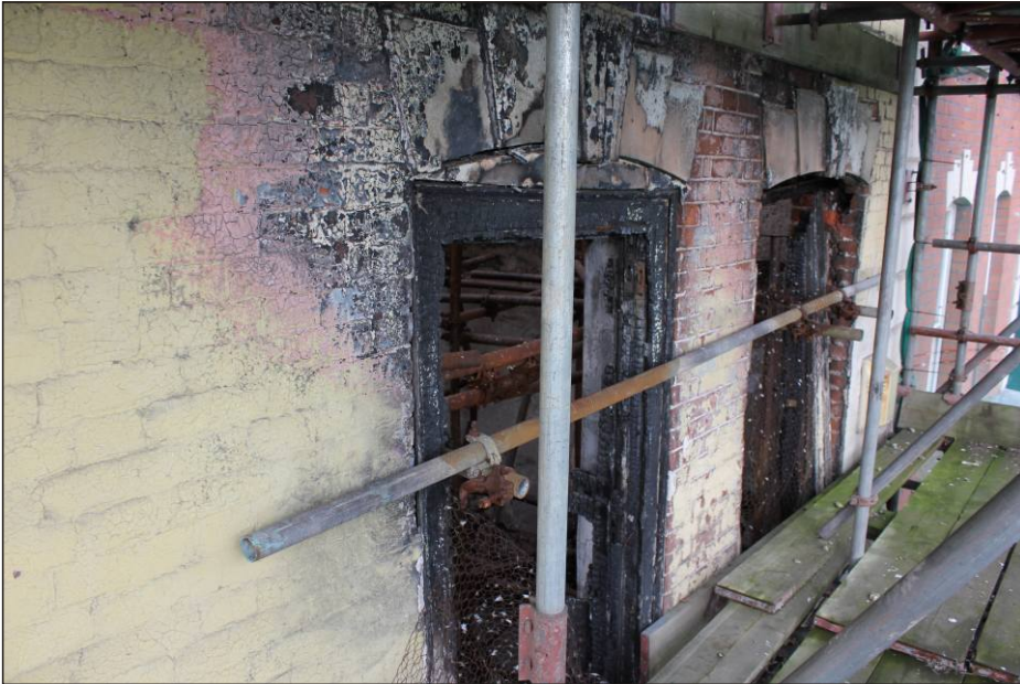
Plate 4: The first floor of the front elevation showing brickworks and window openings, viewed from the south.
