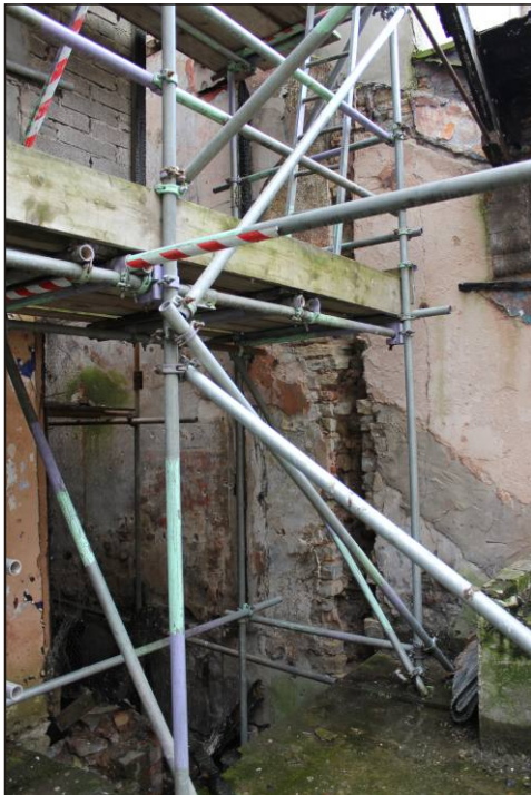
Plate 18: Scars of the roof and stairs in the west boundary wall, viewed from the north.
