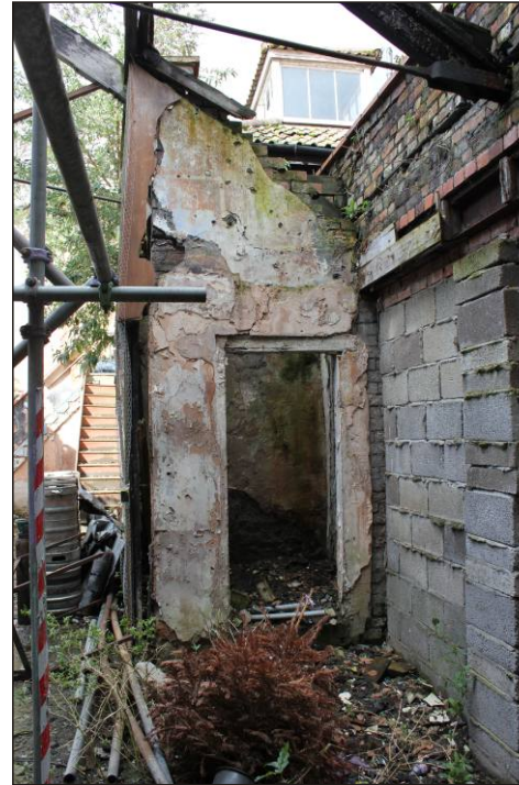
Plate 17: The rear east wall showing inserted and blocked doorway and small outbuilding beyond, viewed from the southeast.
