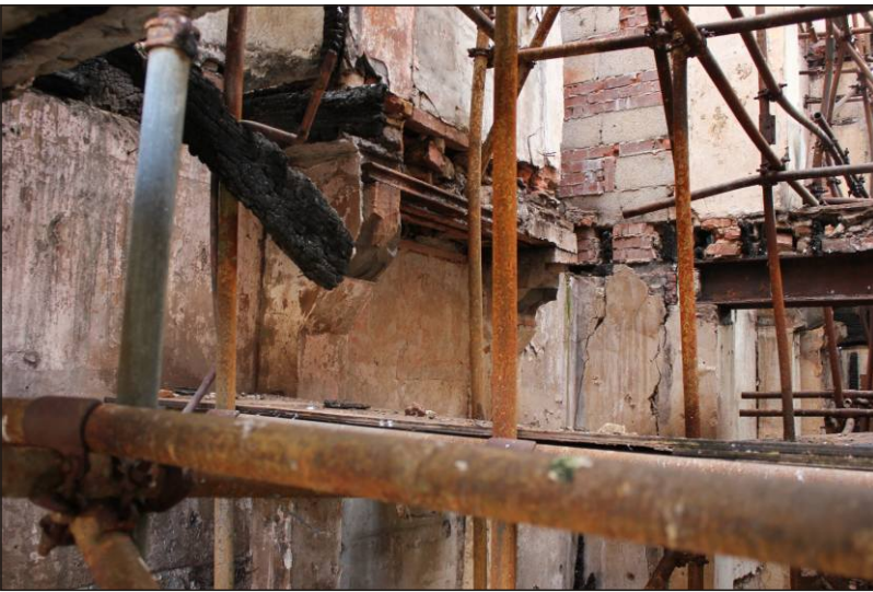
Plate 11: The supports for the first-floor fireplace in the rear room, viewed from the west.
