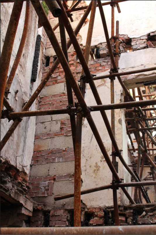
Plate 13: The first-floor partition wall showing joist sockets, inserted doorway and rebuilt masonry, viewed from the northwest.
