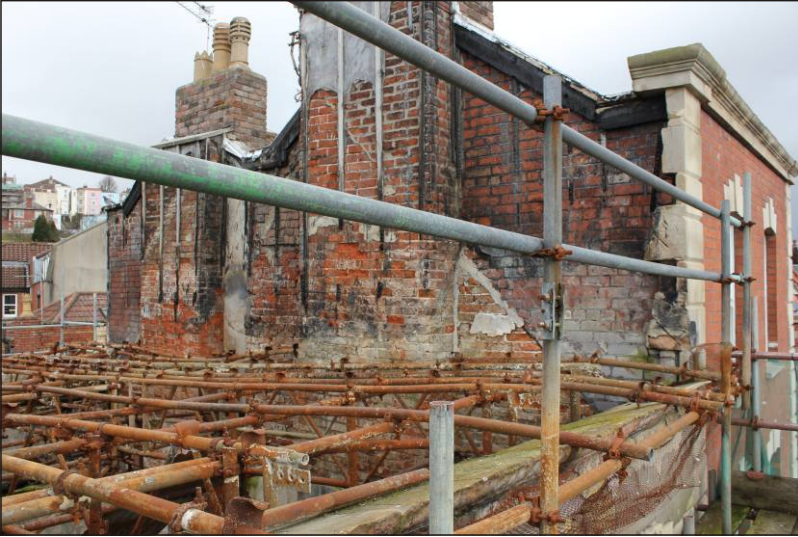
Plate 10: The chimney stacks at roof level, showing the scars of the rooflines and the extended masonry of No. 43, viewed from the south.
