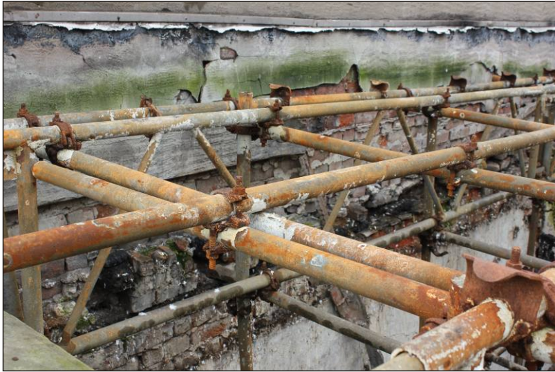
Plate 16: The joist sockets of the second-floor ceiling within the party wall with no. 39, viewed from the east.
