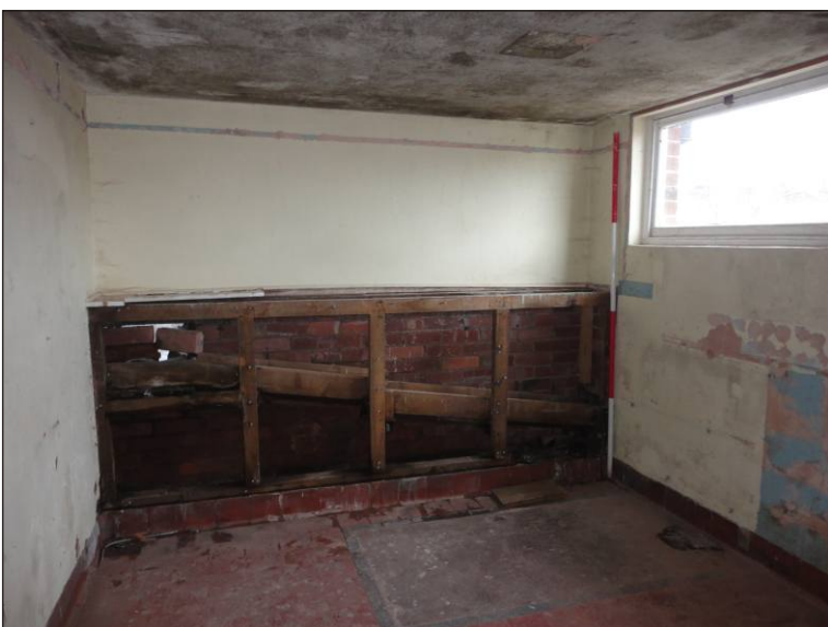
Plate 15: Halford Wing, third floor, drain
