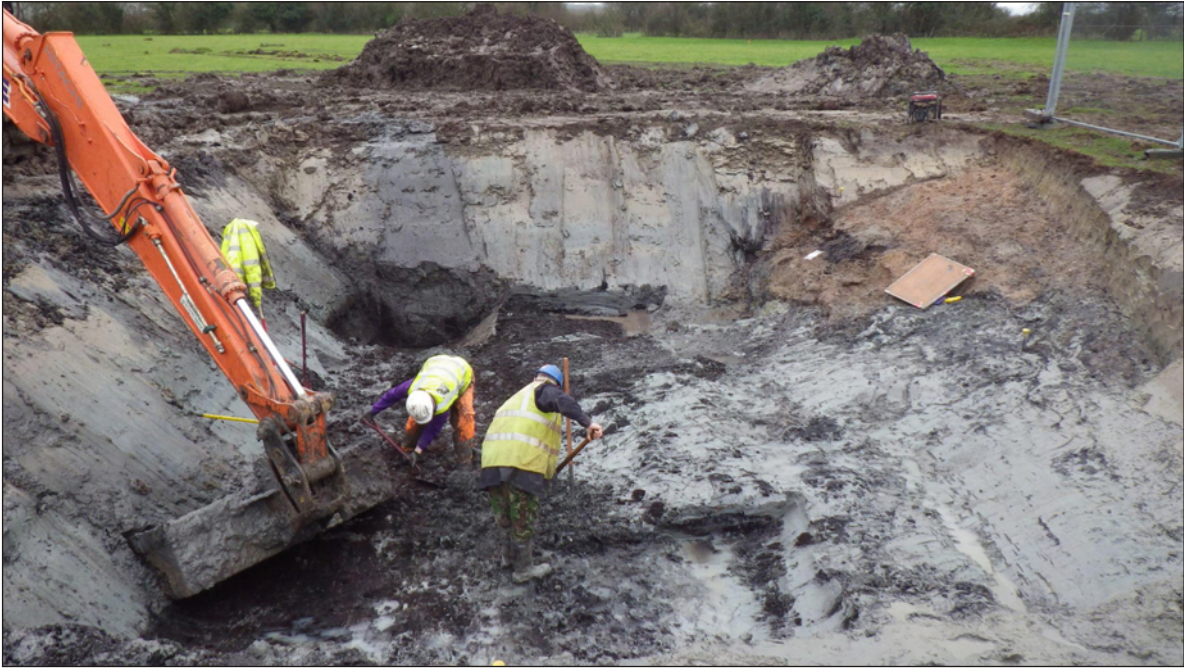
Plate 1: General view of the site, work in progress, viewed from the southeast
