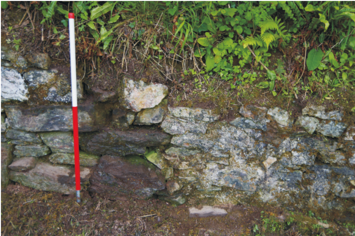
Plate 5: Zone 2, northwest wall, break between block and rubble coursing, viewed from the north. 1m scale
