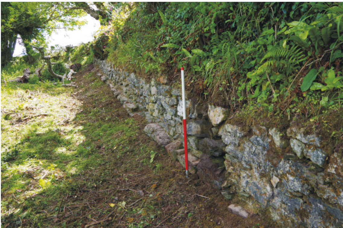
Plate 6: Zone 2, northwest wall, showing stepped coursing at base, viewed from the northwest. 1m scale
