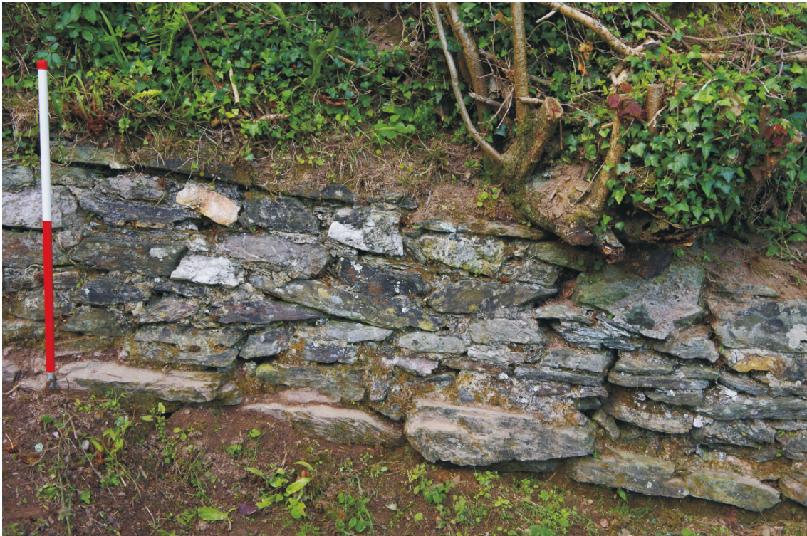
Plate 4: Zone 2, northwest wall, squared block coursing and base step, viewed from the north. 1m scale
