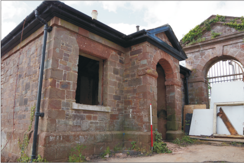
Plate 1: North elevation of the lodge, with the gateway in the background, looking from the northeast (1m scale)
