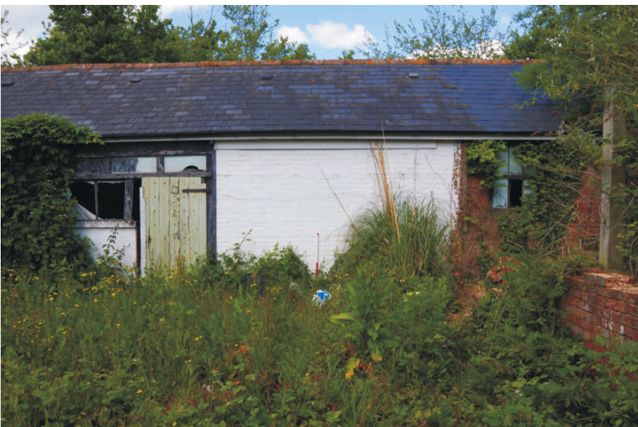
Plate 12: The east elevation of the western building in the U range, looking west (1m scale)
