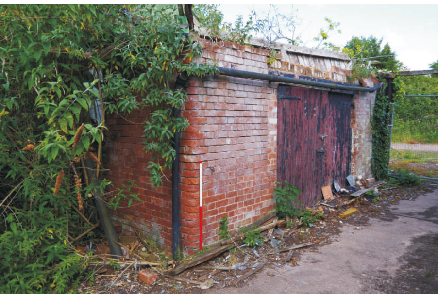
Plate 15: The building at the north end of the western building in the U range, looking northwest (1m scale)
