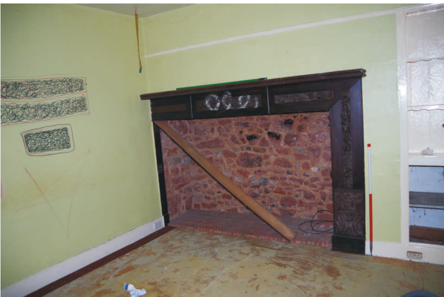
Plate 6: The fireplace on the ground floor of the house, looking northeast (1m scale)
