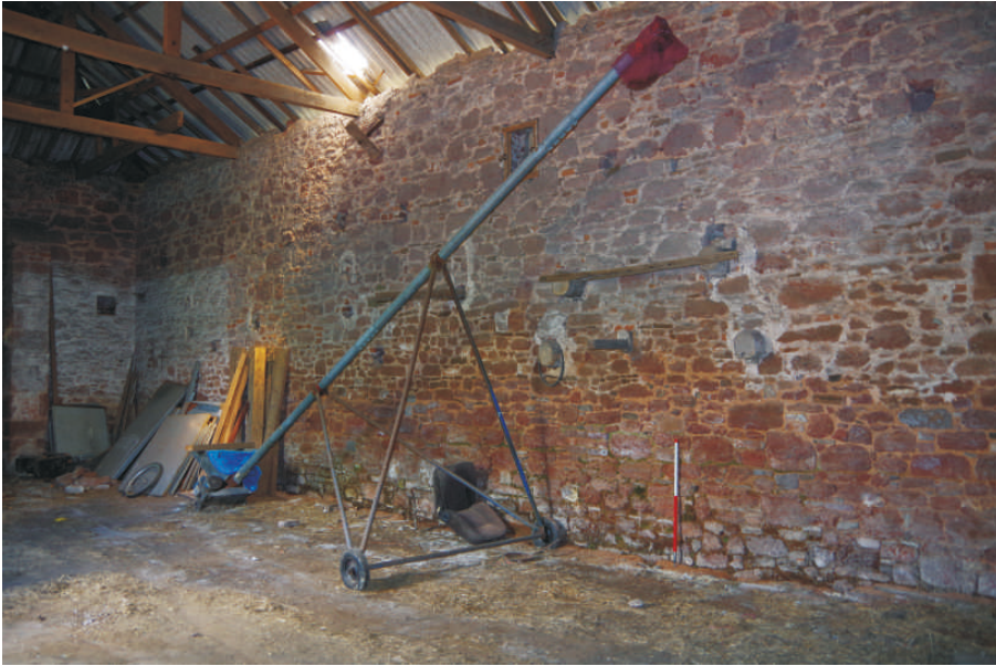
Plate 27: Holes for beams in the northern end of the old barn, looking northeast (1m scale)
