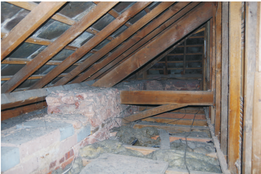
Plate 8: The top of the wall and roof trusses in the house, looking northeast
